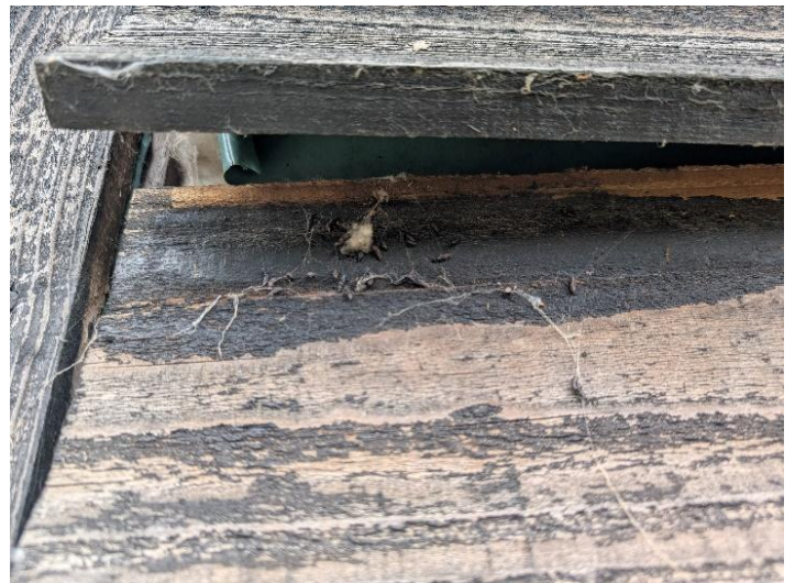
Figure 8: Bat droppings below lifted timber weatherboarding (B5)
