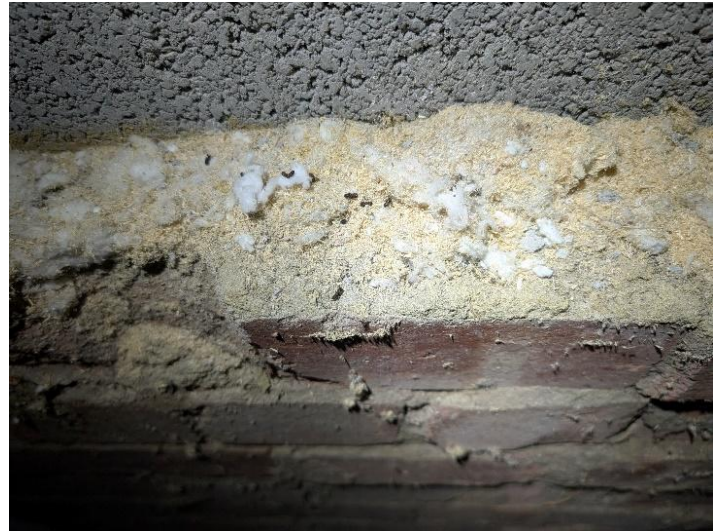
Figure 4: Bat droppings below timber fixed to wall in B1
