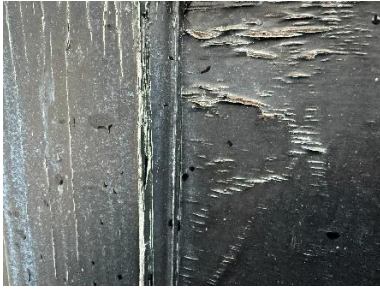
Figure 2 – Decay & poor decorations to timber.
