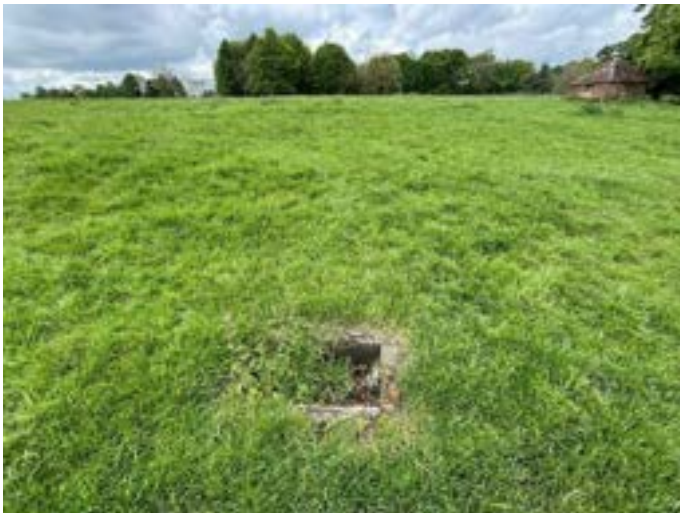
Figure 11: View of further disused drainage features facing south-west.
