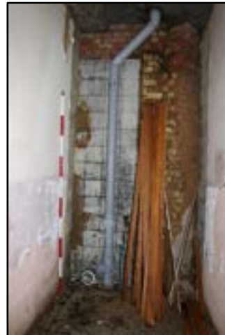
DP 104 Evidence of tiles within a cupboard in the north wing, taken from the south-east
