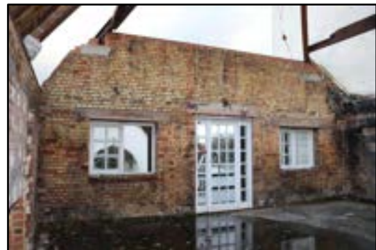
DP 124 Surviving upper structure to the south-east range, taken from the south
