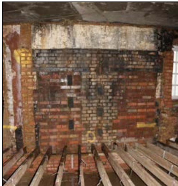
Proposal 5: Area of proposed new doorway showing extensive disturbance in the brickwork (DP94)
