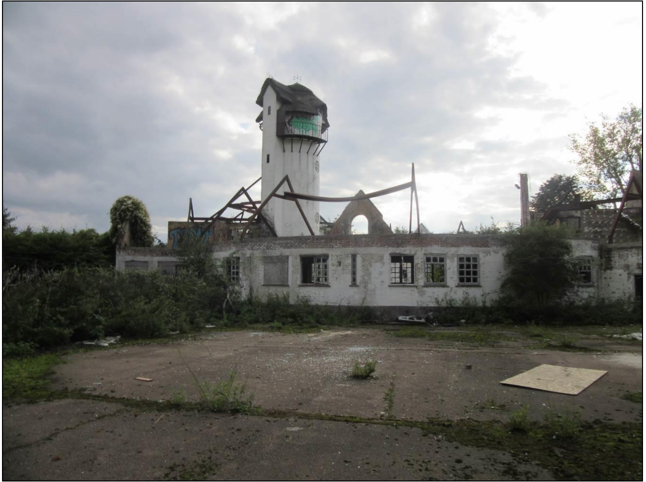
Photograph K – Showing the condition of the Listed Building.
