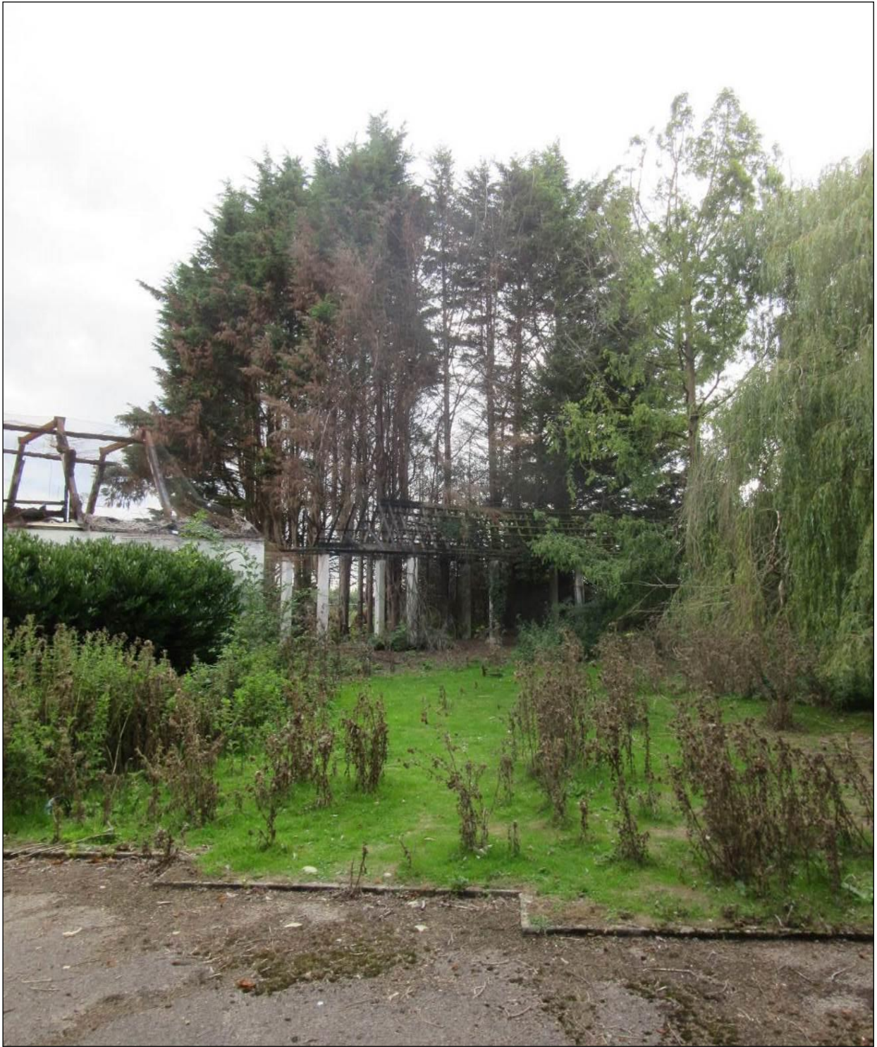
Photograph F – Showing fire damage to G1.
