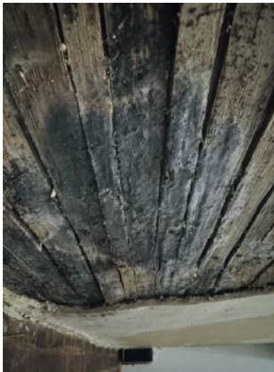
FAILURE OF LATH & PLASTER CEILING DUE TO WATER PENETRATION
