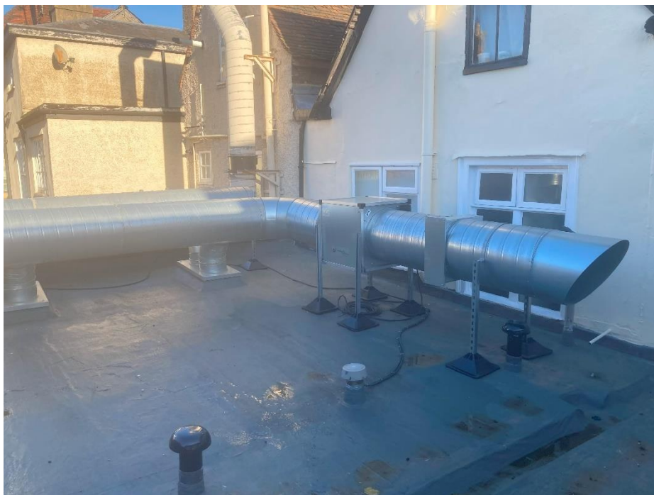
Figure 7 Kitchen extract intake
