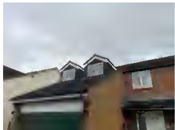
Photograph 6. Showing the intact dormer windows including the lead flashing and barge board. Showing the slightly lifting soffit.
