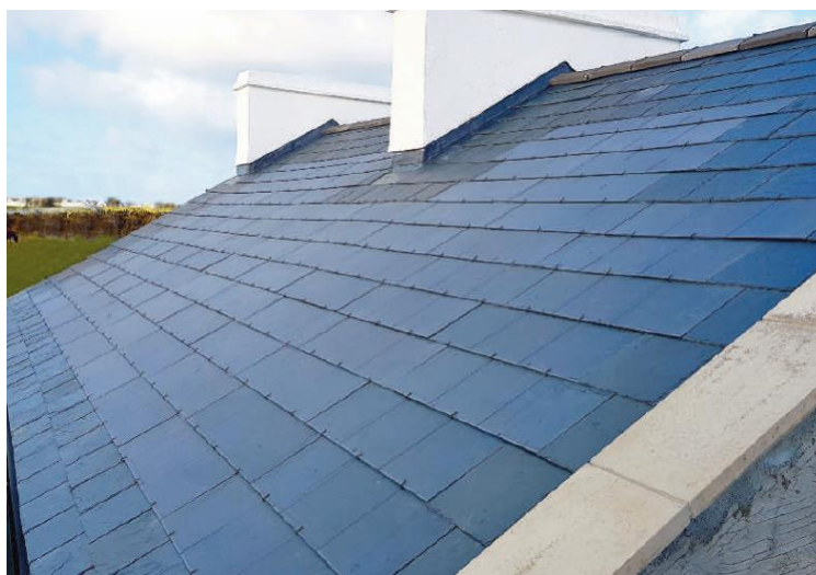
Figure 5: PV Slate System
