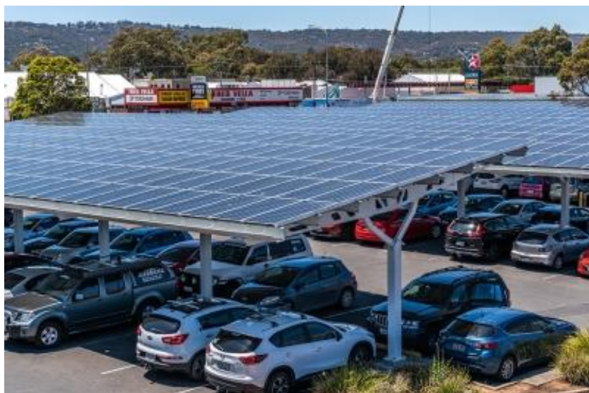
Figure 4: Example Car Park Solar PV Array
