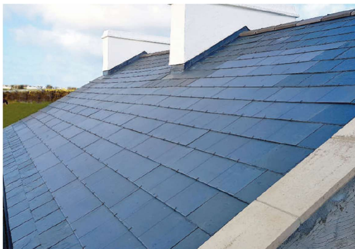
PV Slate System
