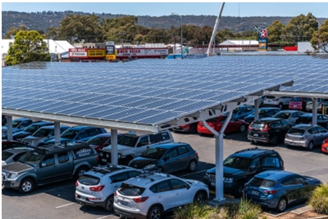
Example Carpark Solar PV Array
