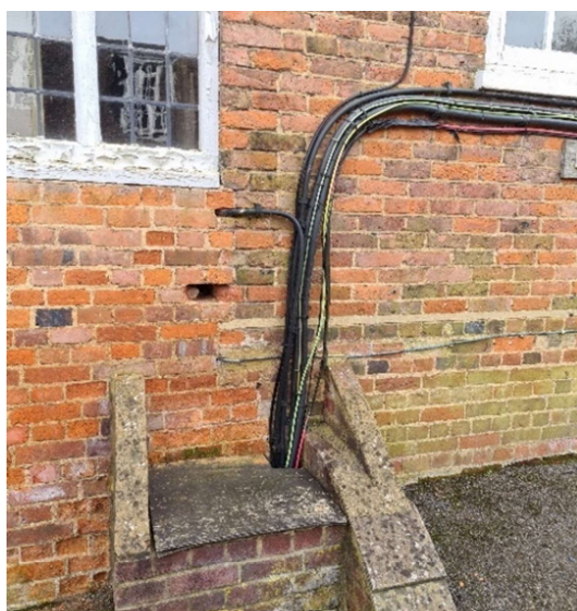
Outgoing submains on façade of building
