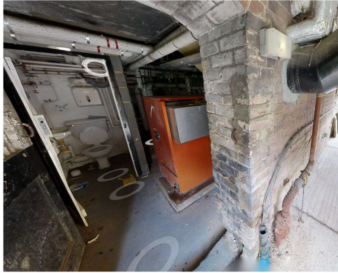
Teaching Block – Basement Gas Fired Boiler
