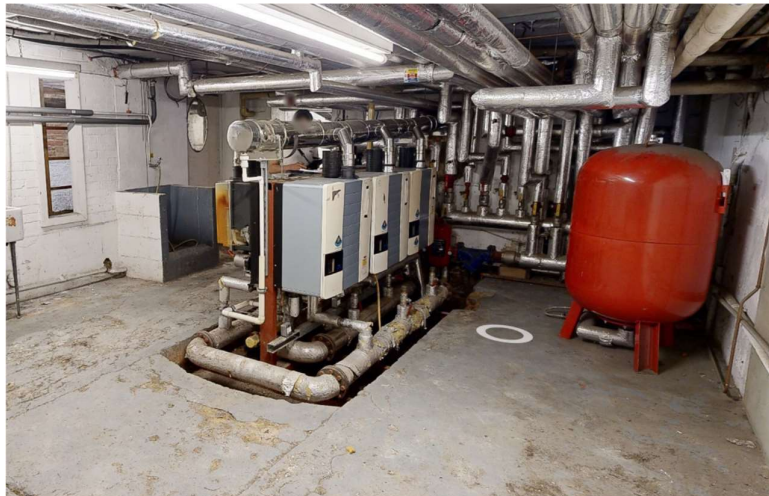
Main Building – Basement Gas Fired Boilers
