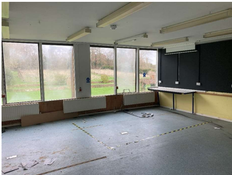
Existing luminaires within the school building.
