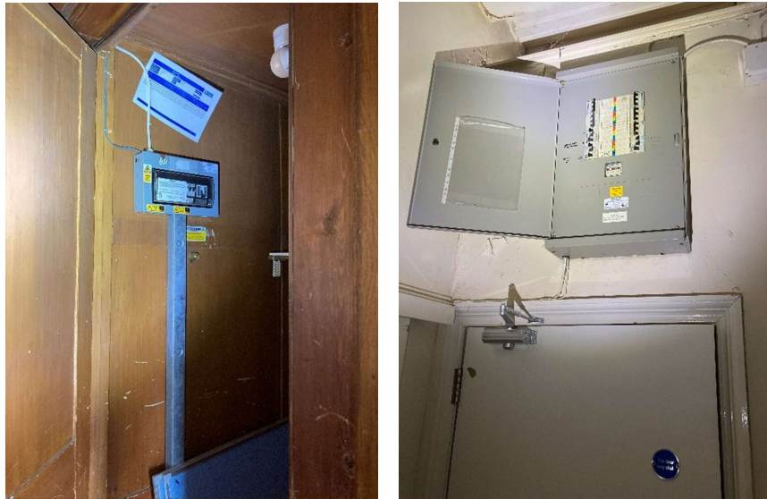
Old distribution boards located within the listed building
