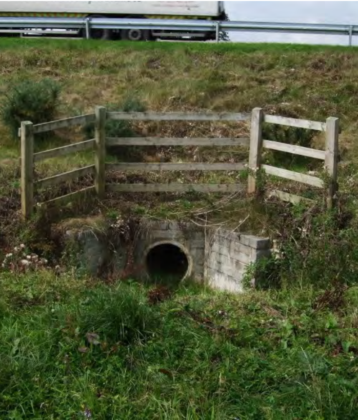
▲ Tunnels under roads help prevent mammal deaths due to traffic
