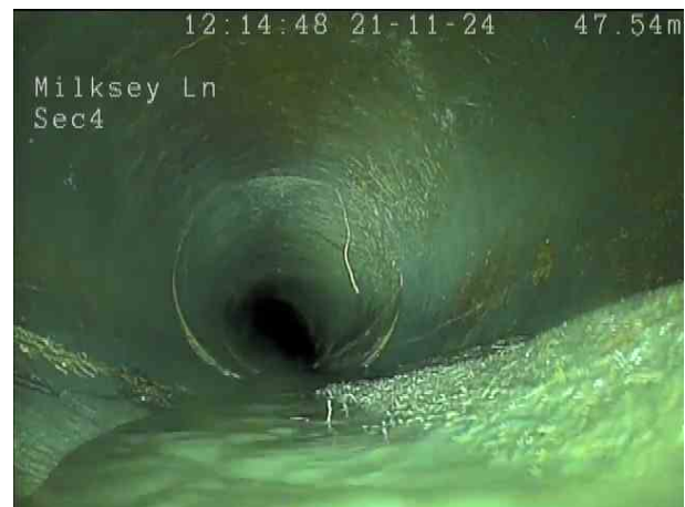
6d0965e6-bcb2-4139-864b-f7b8d1967d73.png, 00:05:12, 47.50 m Roots, mass at joint, 10% cross-sectional area loss, change
