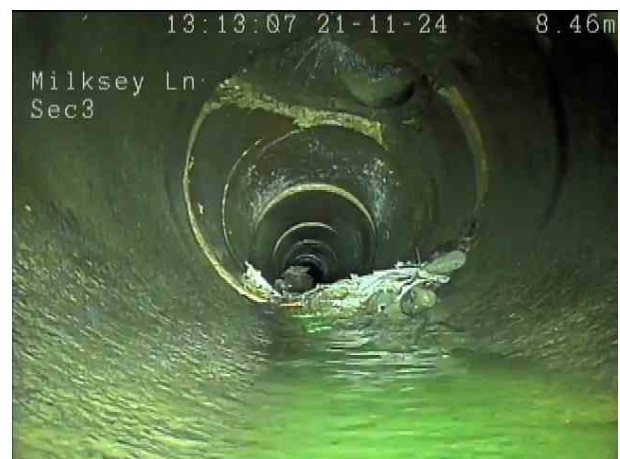
b65f7ef7-e37d-4f68-8e9d-51e517b19886.png, 00:01:07, 8.90 m Connection defective, connecting pipe is damaged at 1 o'clock,
