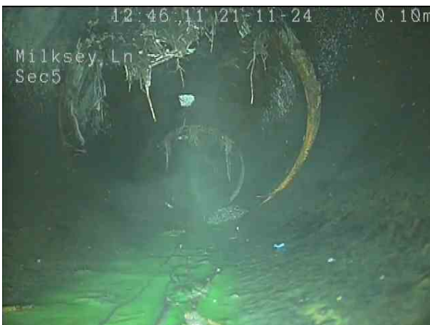
d75d1e6c-e1ee-4a24-8fba-f6bf955d0141.png, 00:00:08, 0.50 m Roots, mass at joint, 10% cross-sectional area loss, start
