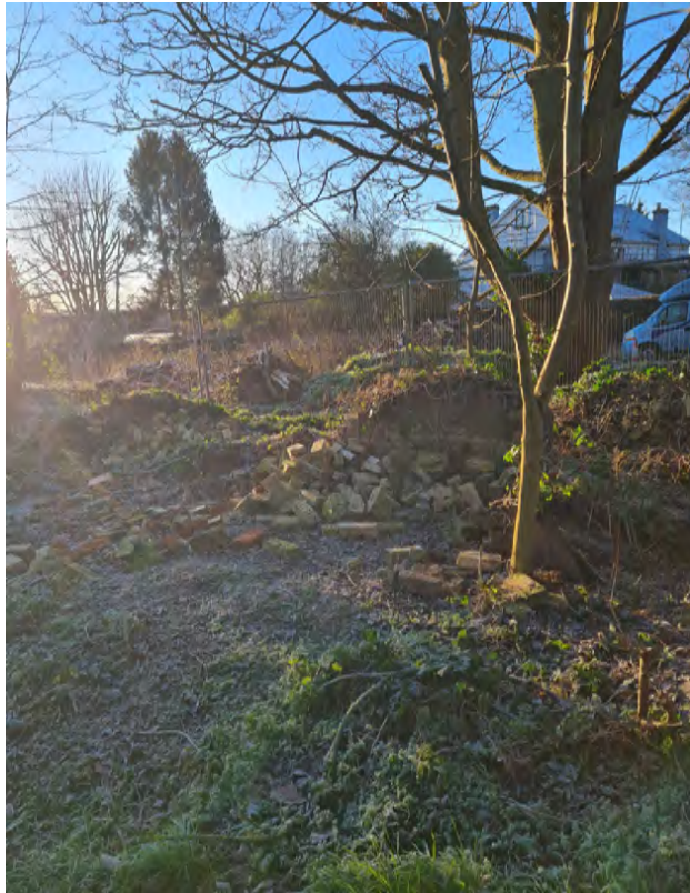
Photograph 3: Wall remains and building rubble in the centre of the Site.
