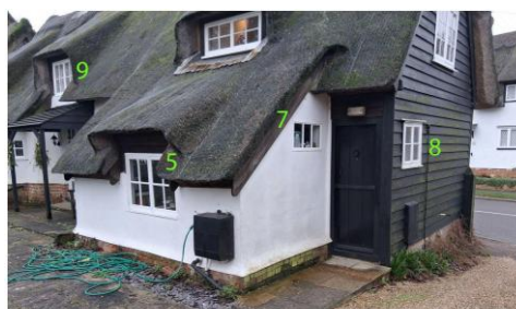
Rear_03: Kitchen (5 & 7), middle bedroom (9) and side of house (8) windows to be replaced.
