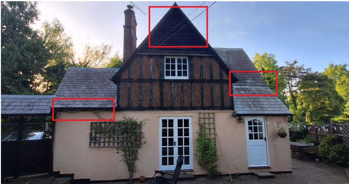
Photograph 8: Potential roost features identified on the eastern aspect, Building A. Recommended view for survey.
