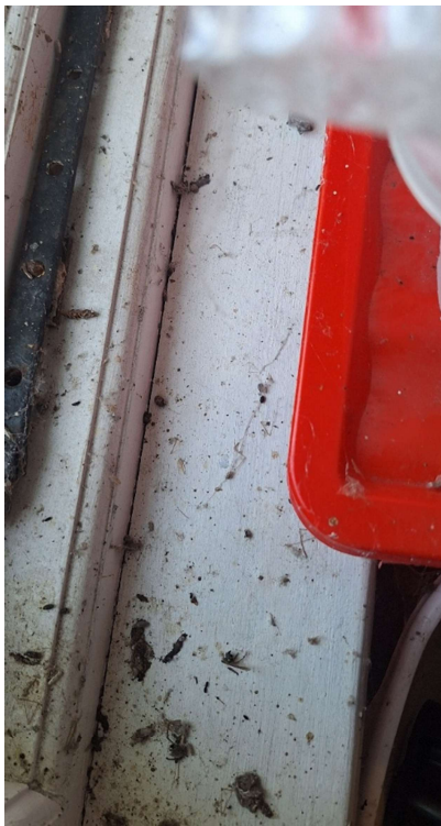
Photographs 6. Mouse droppings, Building B
