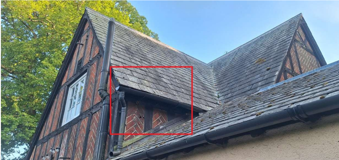
Photograph 12: Hole in brickwork on the northern aspect of the upper storey. Recommended view for survey.
