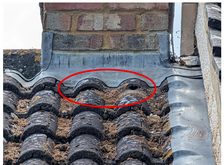
Figure 4: Northeast elevation roof. Potential exit/entry hole and roosting feature under tiles
