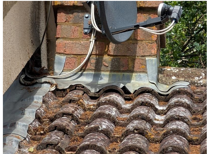
Figure 6: Southwest elevation of single storey room. Potential roosting feature under flashing and lifted tiles
