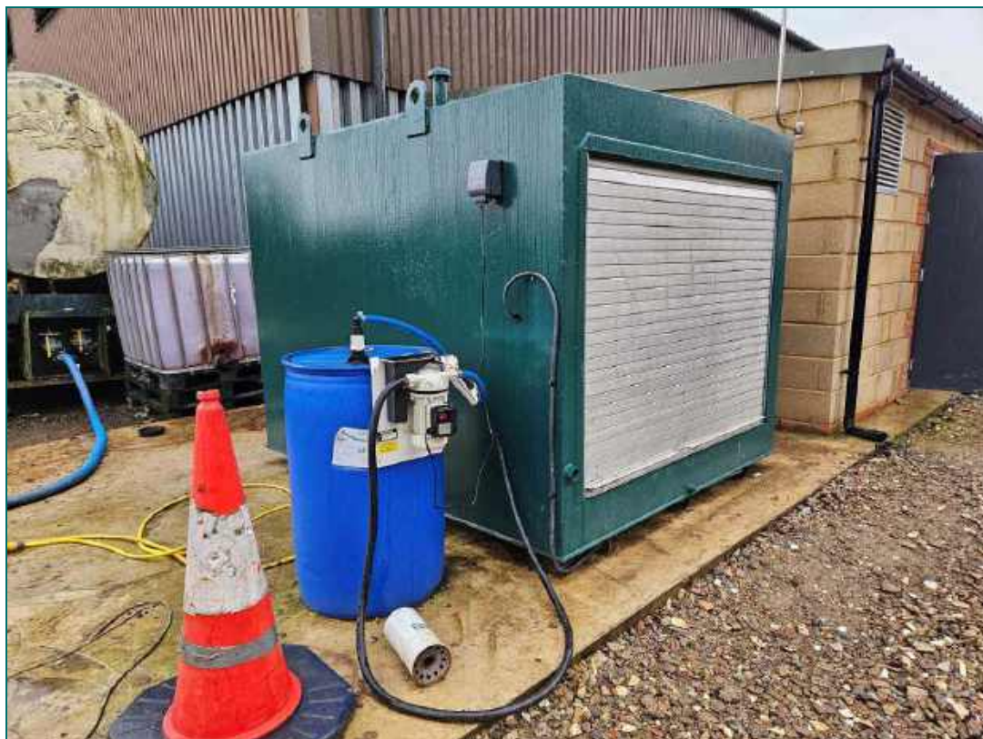
Photograph 5: Fuelling Facility at Munches Farm.
