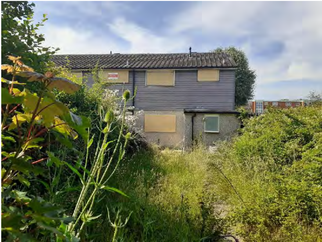
Plate 5: Rear garden of No. 5 Newells, which is overgrown and derelict, taken from the north.
