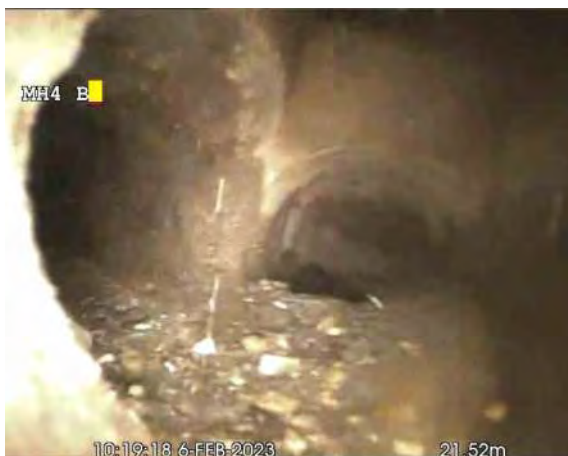
51395fd3-0329-4168-beb3-8c67e194c290.jpg, 00:01:44, 21.62 m Junction at 9 o'clock, 100mm dia
