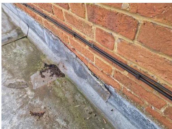
11. Poor flashing detail
