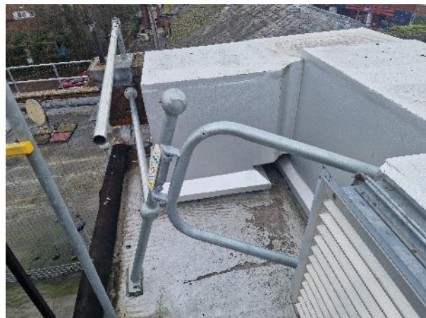
24. Defective edge protection
