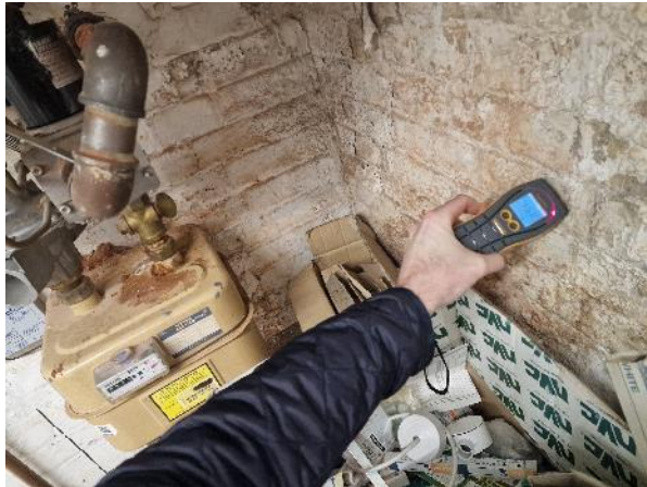
19. Penetrating moisture ingress at basement level
