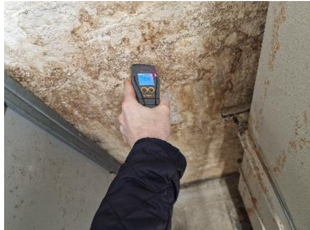
20. Penetrating moisture ingress at basement level
