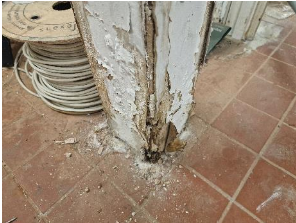
21. Timber decay to supporting post
