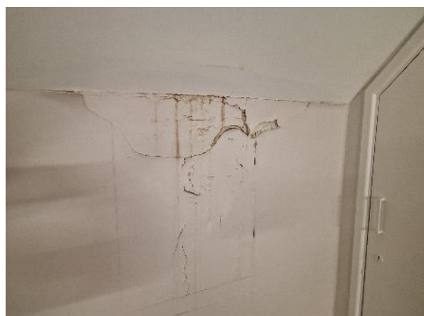
12. Water ingress from main roof
