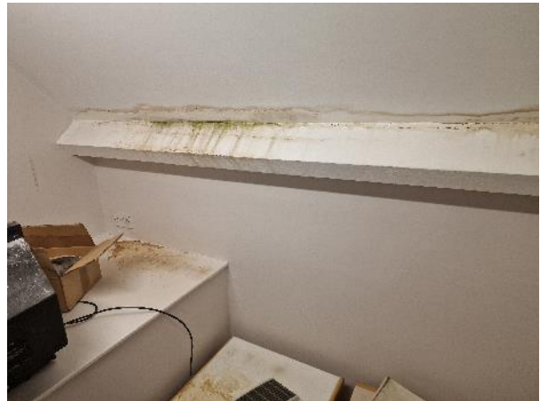
14. Water ingress from main roof
