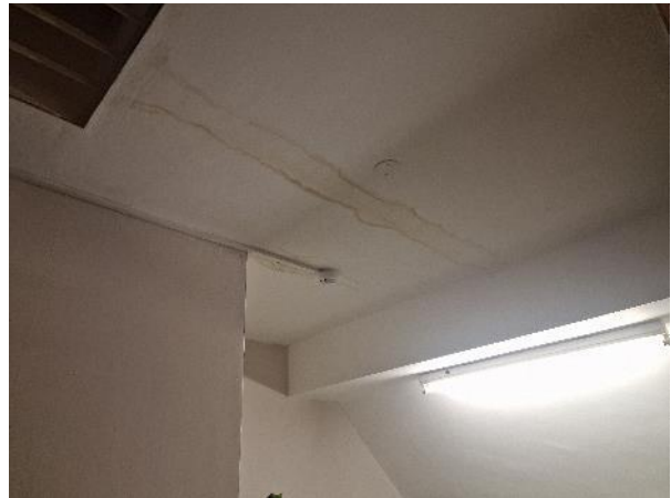
16. Water ingress from central crown
