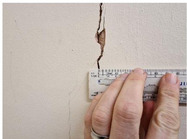
18. Cracking at first floor level
