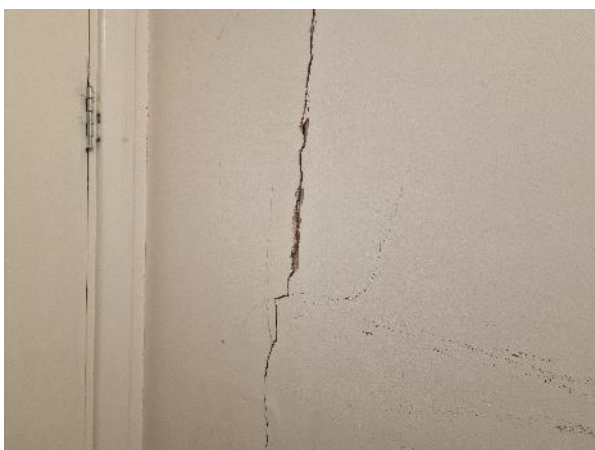
17. Cracking at first floor level
