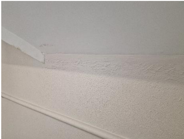
13. Water ingress from main roof
