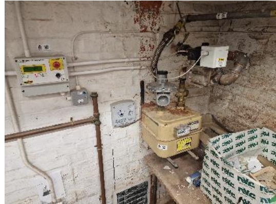
Photograph K – Damp ingress at basement level
