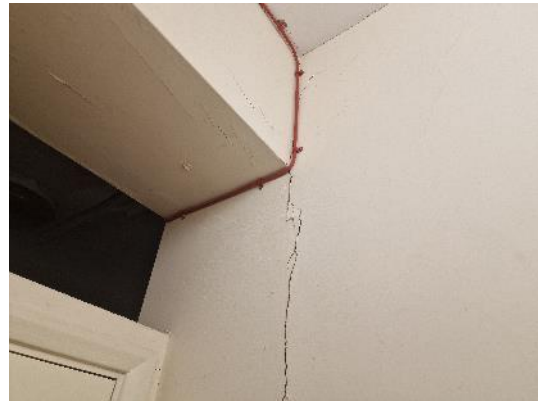
Photograph I – Evidence of cracking at first floor level
