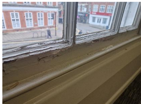
Photograph J – Water ingress emanating from window frames
