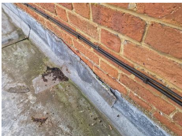
11. Poor flashing detail
