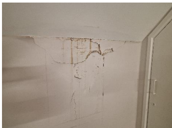
12. Water ingress from main roof
