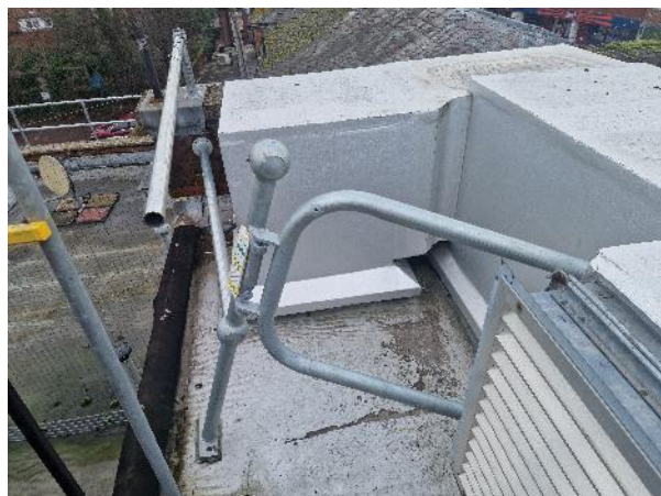
24. Defective edge protection
