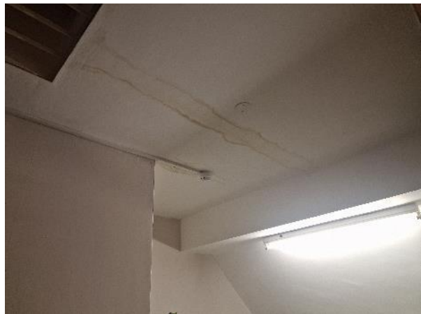
16. Water ingress from central crown
