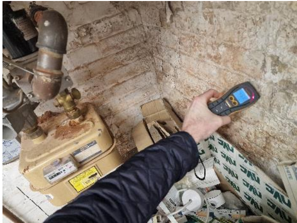
19. Penetrating moisture ingress at basement level
