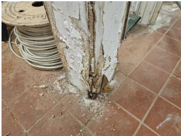
21. Timber decay to supporting post
