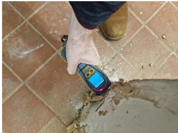
22. Timber decay to supporting post
