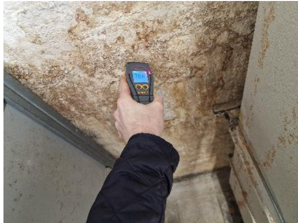
20. Penetrating moisture ingress at basement level
