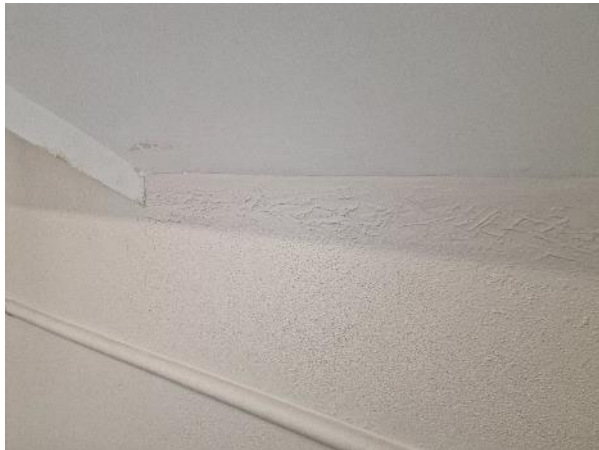
13. Water ingress from main roof
