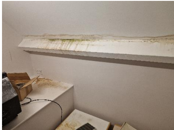
14. Water ingress from main roof
