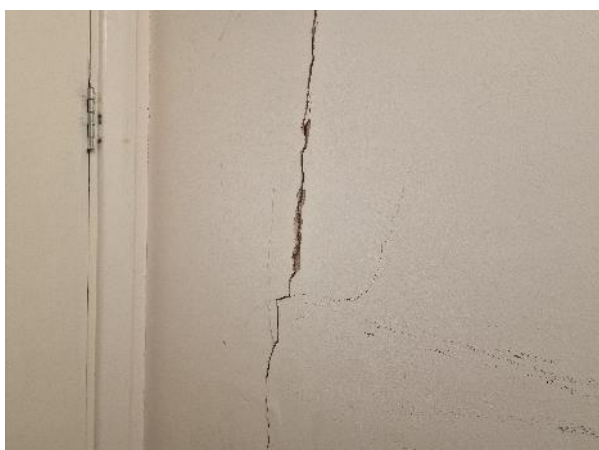
17. Cracking at first floor level
