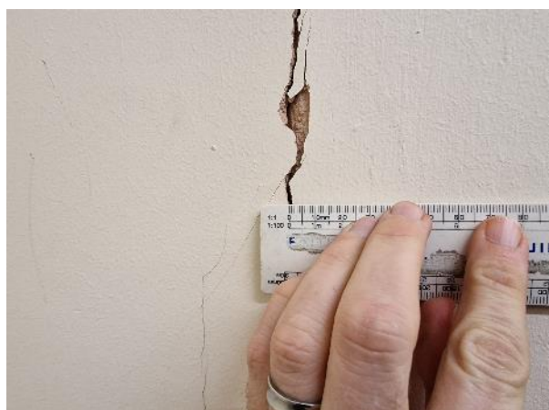
18. Cracking at first floor level
