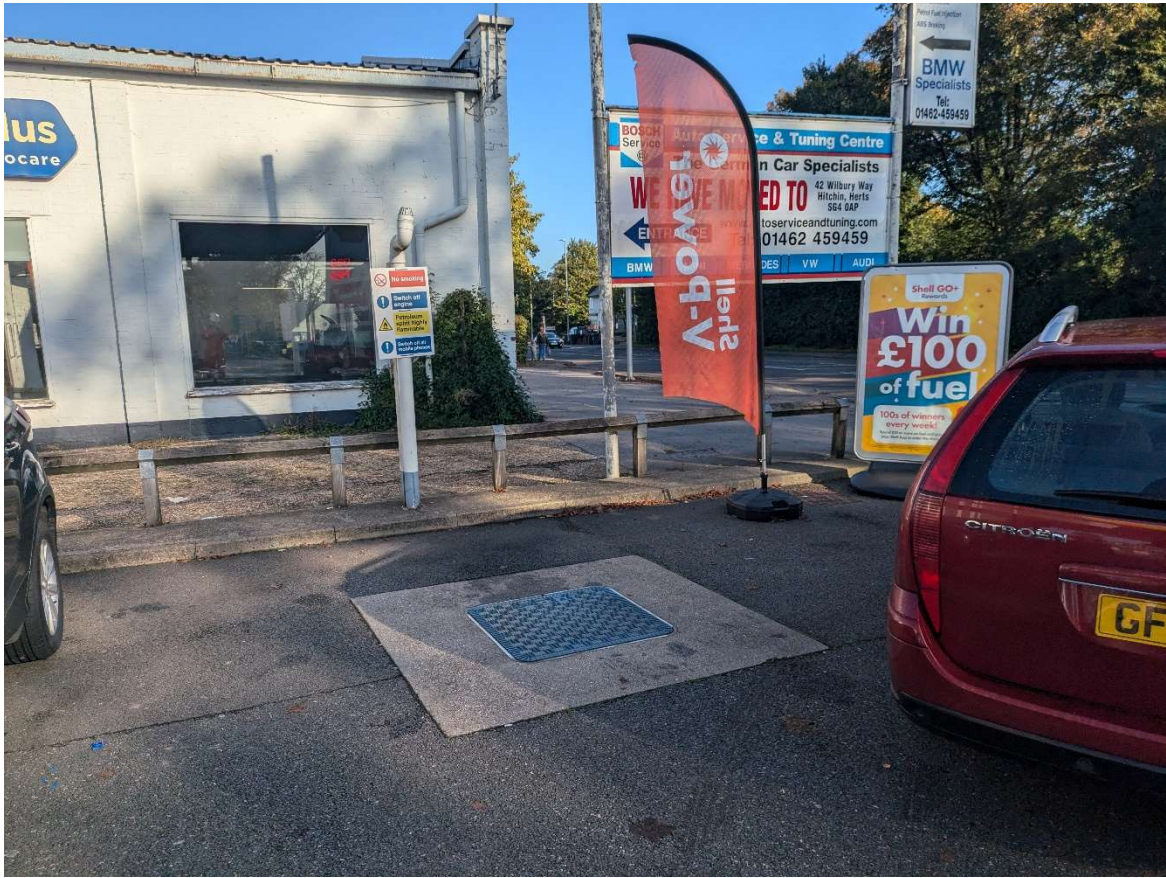
Main interceptor located northeast of the Site
