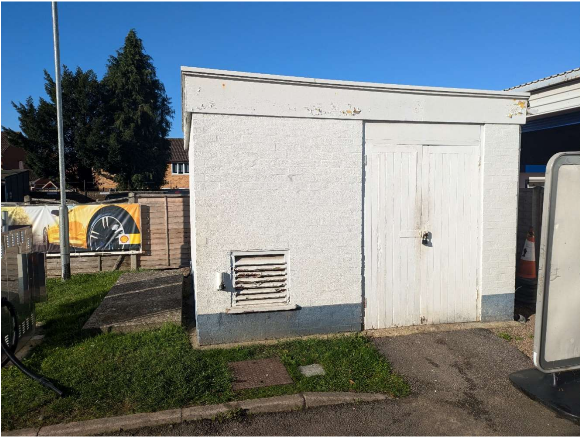
Car Wash Plant room
