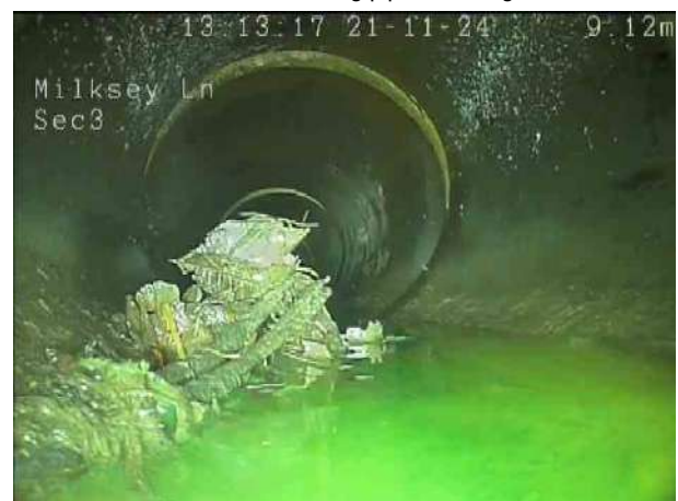
035ad4f6-410a-4705-9adf-9434a6787c09.png, 00:01:16, 9.20 m Settled deposits, other, 10% cross-sectional area loss, Leaves
