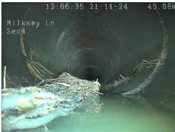
2ac8cc72-35a9-48b6-8983-1817bcbaa44d.png, 00:04:03, 45.30 m Roots, mass at joint, 15% cross-sectional area loss, start
