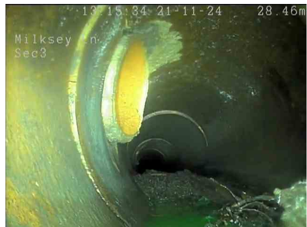
c149e879-bbbf-4cb7-8b94-35e5cef6f891.png, 00:03:34, 28.70 m Connection defective, connecting pipe is intruding at 9 o'clock,
