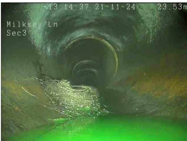
f4683594-3657-44ac-96e9-ee69abbc467a.png, 00:02:37, 23.80 m Roots, mass, 10% cross-sectional area loss, start
