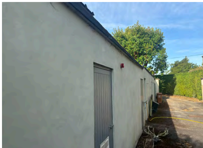
Image 5 - Lack of soffits and fascias.
