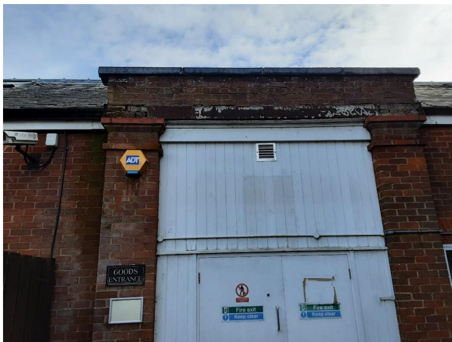
Photograph 9: Cracks in brickwork on northern aspect of Radcliffe House
