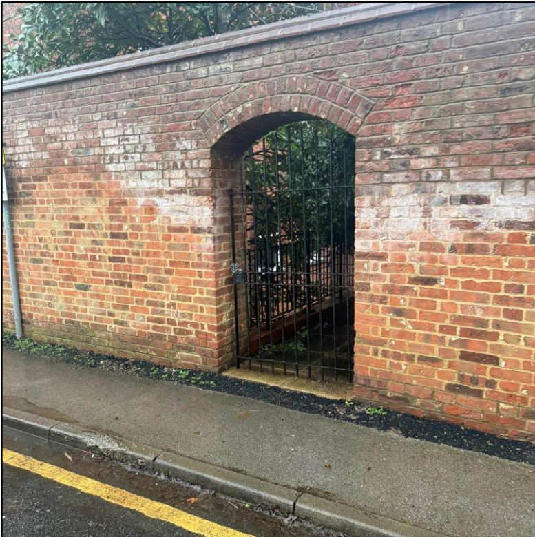
Figure 5: January 2026 photograph showing the current condition of the archway entrance though the site boundary brick wall along Old Charlton Road
