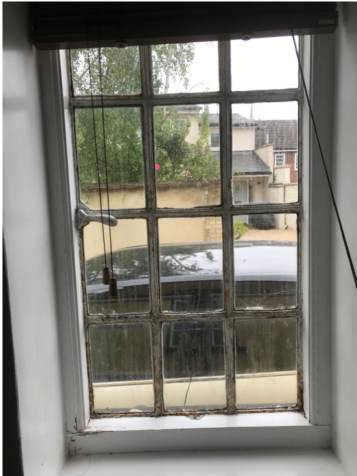
Picture 11: Single casement ground floor entrance hall window, internal (painted shut)
