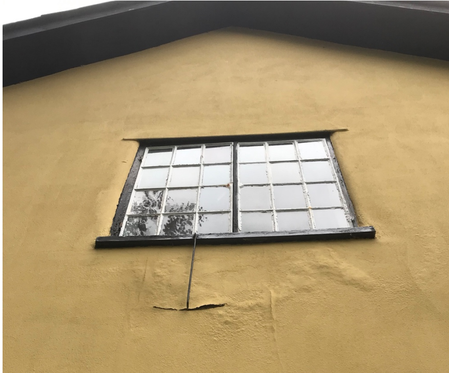
Picture 1: Damage to render caused by traditional window hook under first floor main bedroom window to rear
