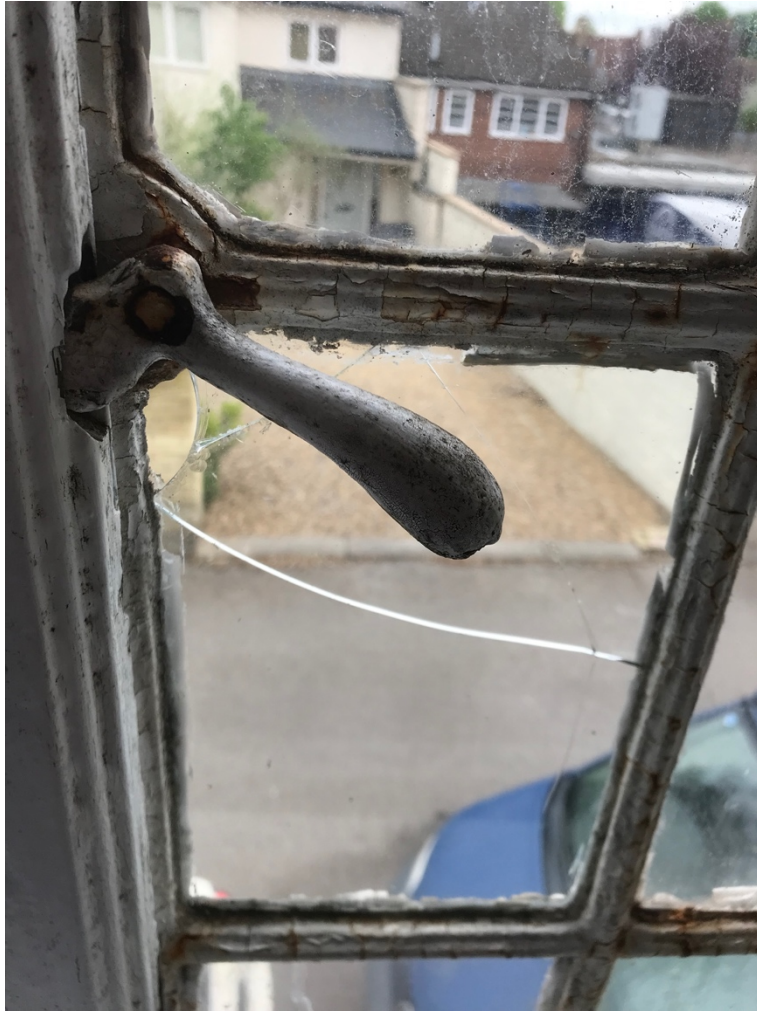
Picture 14: First floor double casement bathroom, cracked pane
