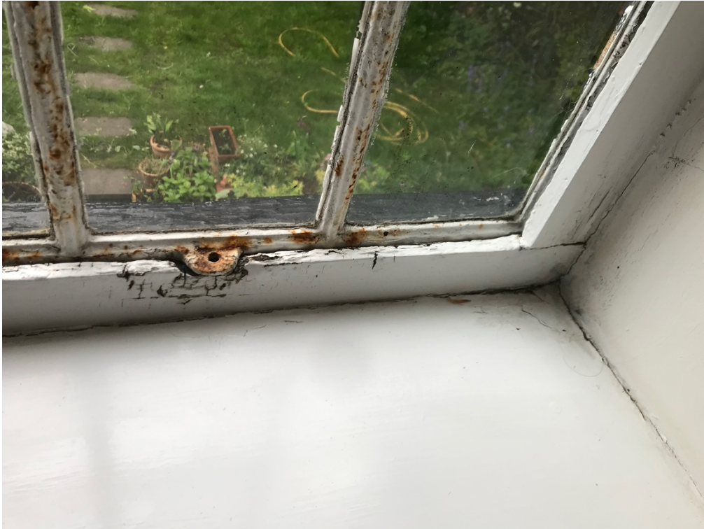
Picture 18: First floor main bedroom double casement cracking and rot in timber frame
