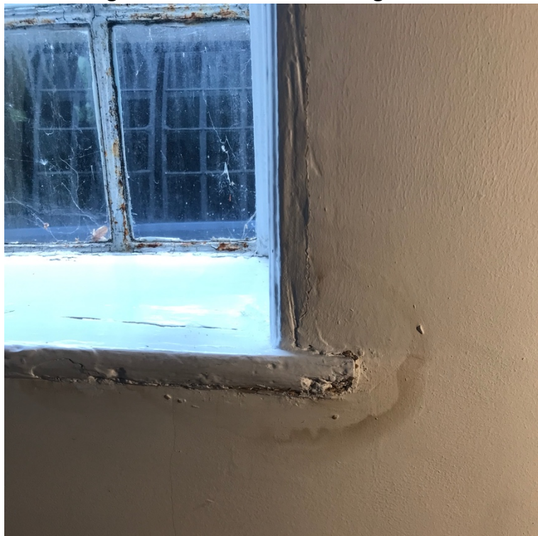
Picture 2: Water damage to internal wall due to condensation run off from double casement ground floor window in living room
