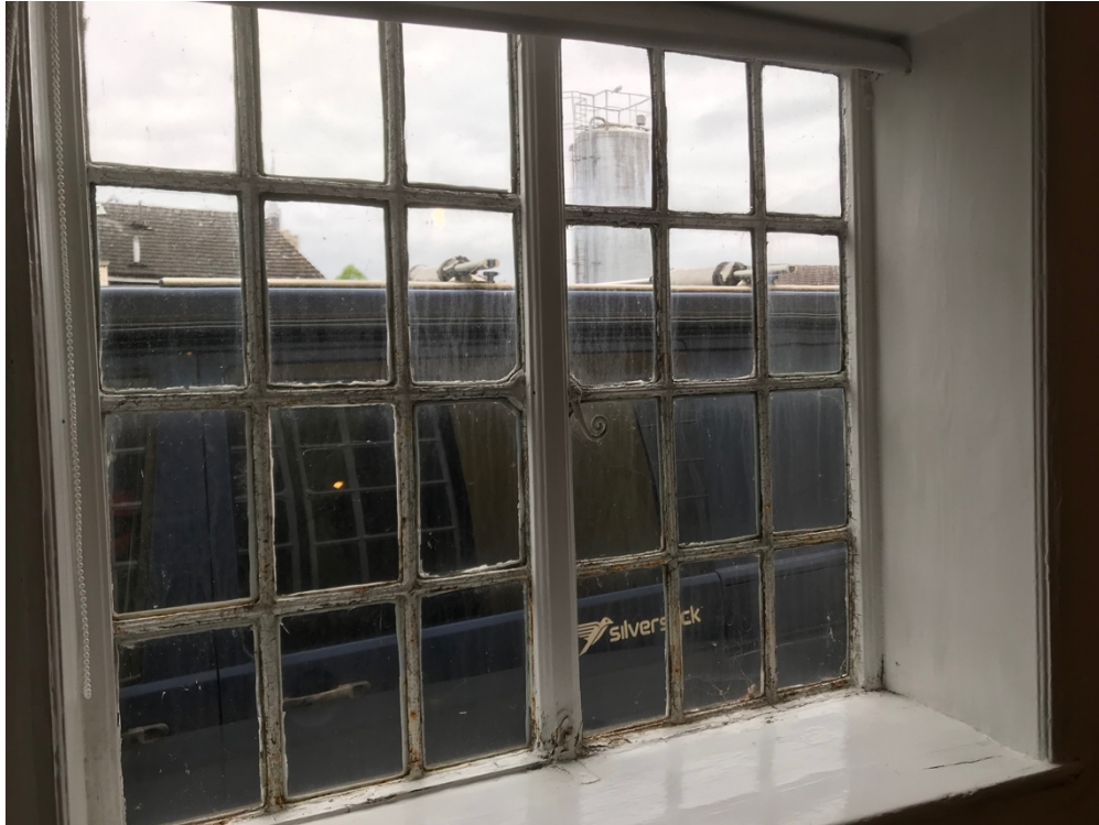
Picture 10: Double casement ground floor living room window internal (painted shut)
