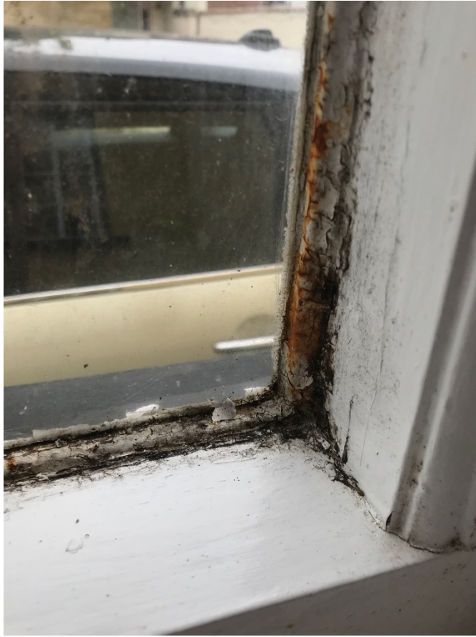
Picture 12: Rotten corners in single casement ground floor entrance hall window
