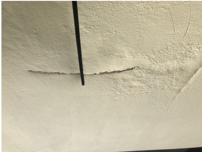
Picture 17: First floor main bedroom double casement, window hook causing damage to render
