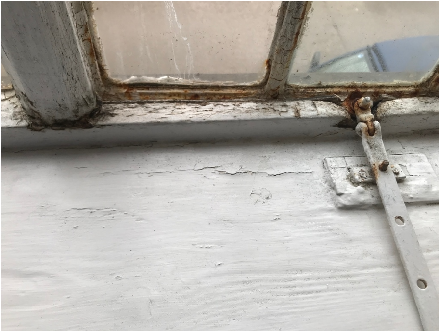
Picture 13: double casement first floor bathroom internal (rot)
