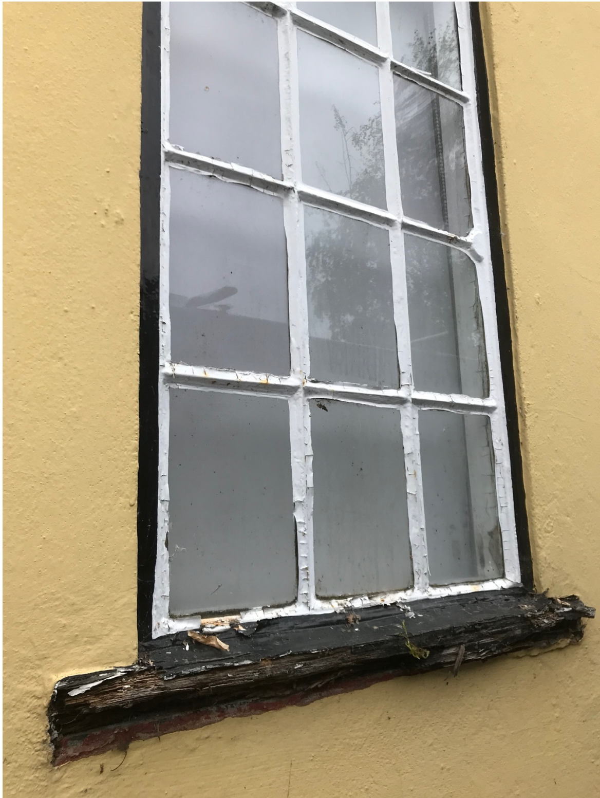
Picture 3: Single casement ground floor living room window - rotten sill. The rotten sill was knocked off by someone walking between vehicles and house and there is now very significant water ingress
