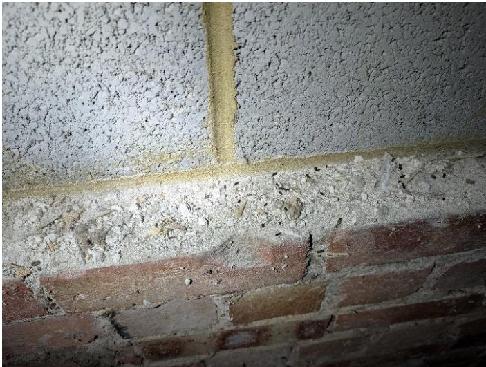
Figure 3: Bat droppings below plasterboard fixed to wall in B1
