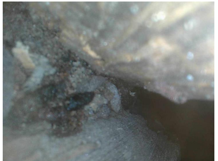
Figure 6: Bat droppings within tenon and mortise joint in B2
