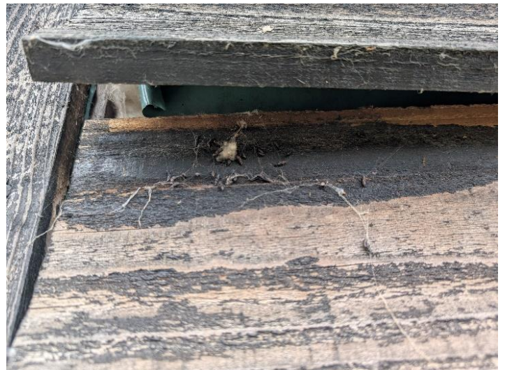
Figure 8: Bat droppings below lifted timber weatherboarding (B5)
