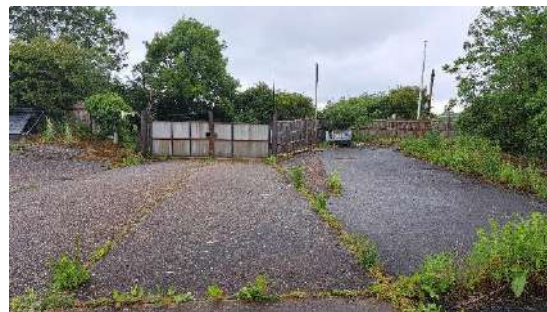
Photo 20 View of Site Access and ruderal vegetation growing through cracks in concrete.
