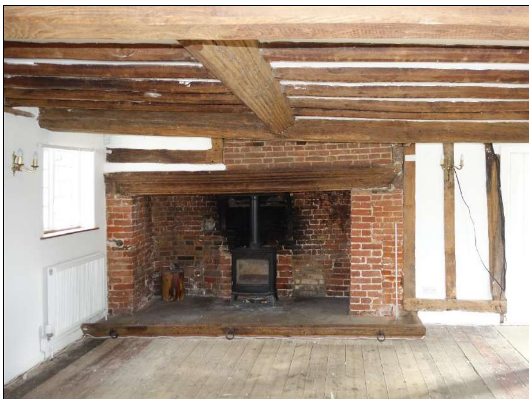
Plate 14: View looking E towards fireplace at E end of sitting room with moulded lintel and roll moulded ceiling beam above
