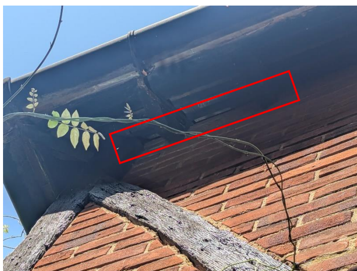
Figure 4: Gaps along eaves (southeast)
