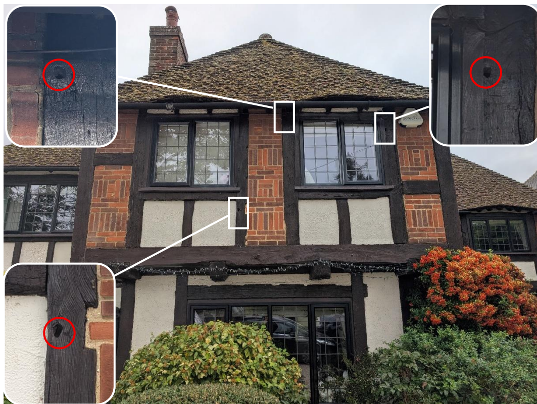
Figure 13: Roosting locations identified by droppings
