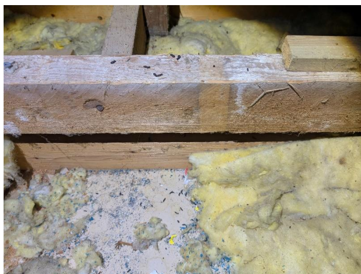
Figure 11: Bat droppings below central ridge beam
