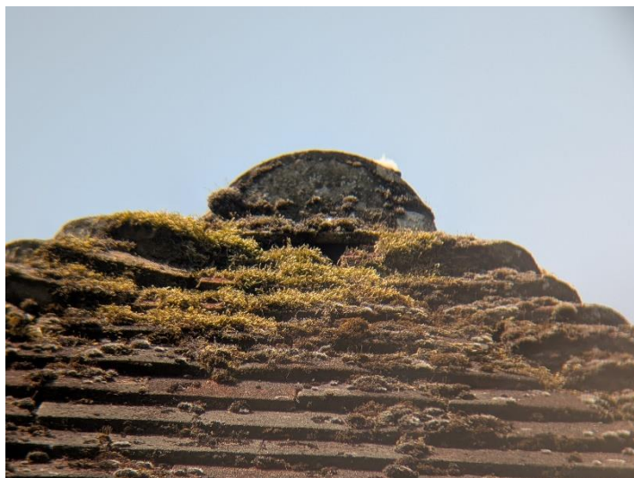
Figure 6: Gap under ridge tile (northeast)
