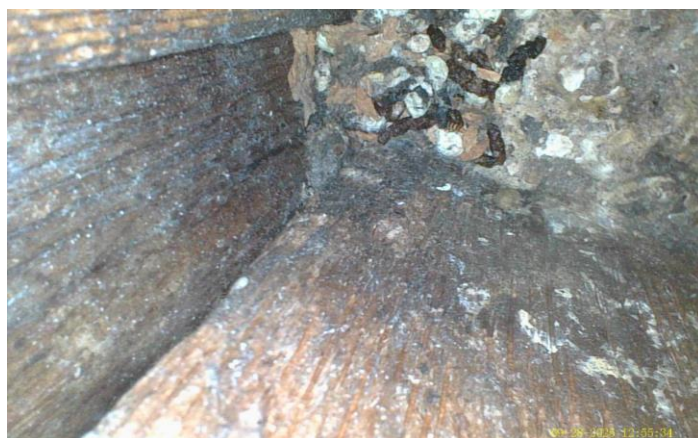
Figure 15: Bat droppings found within timber cavity
