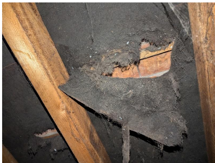
Figure 9: Torn roofing membrane
