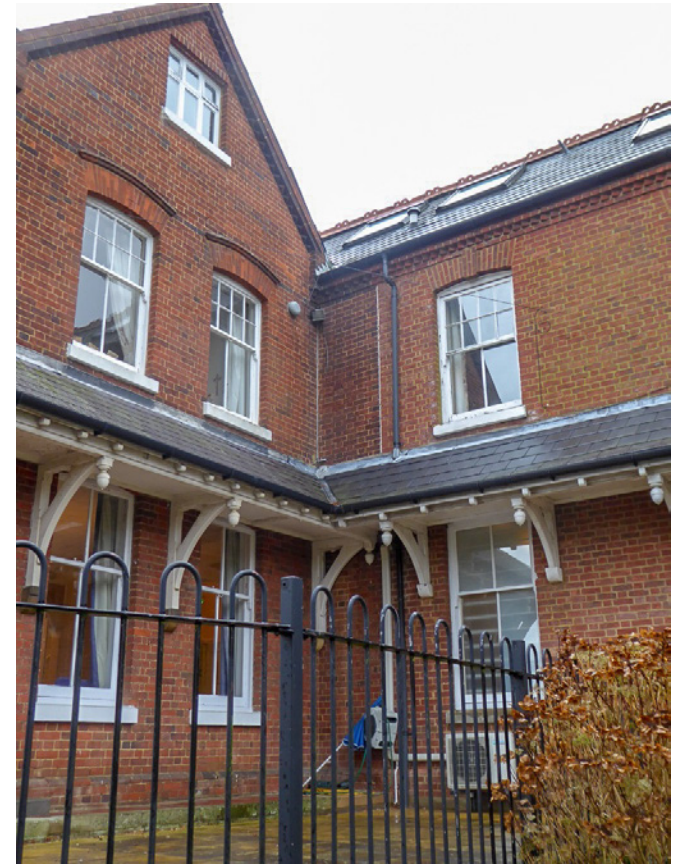
Junction between the original house (left) and the 1980s extension (right). Note the difference in brickwork either side of the expansion joint at first floor level.
