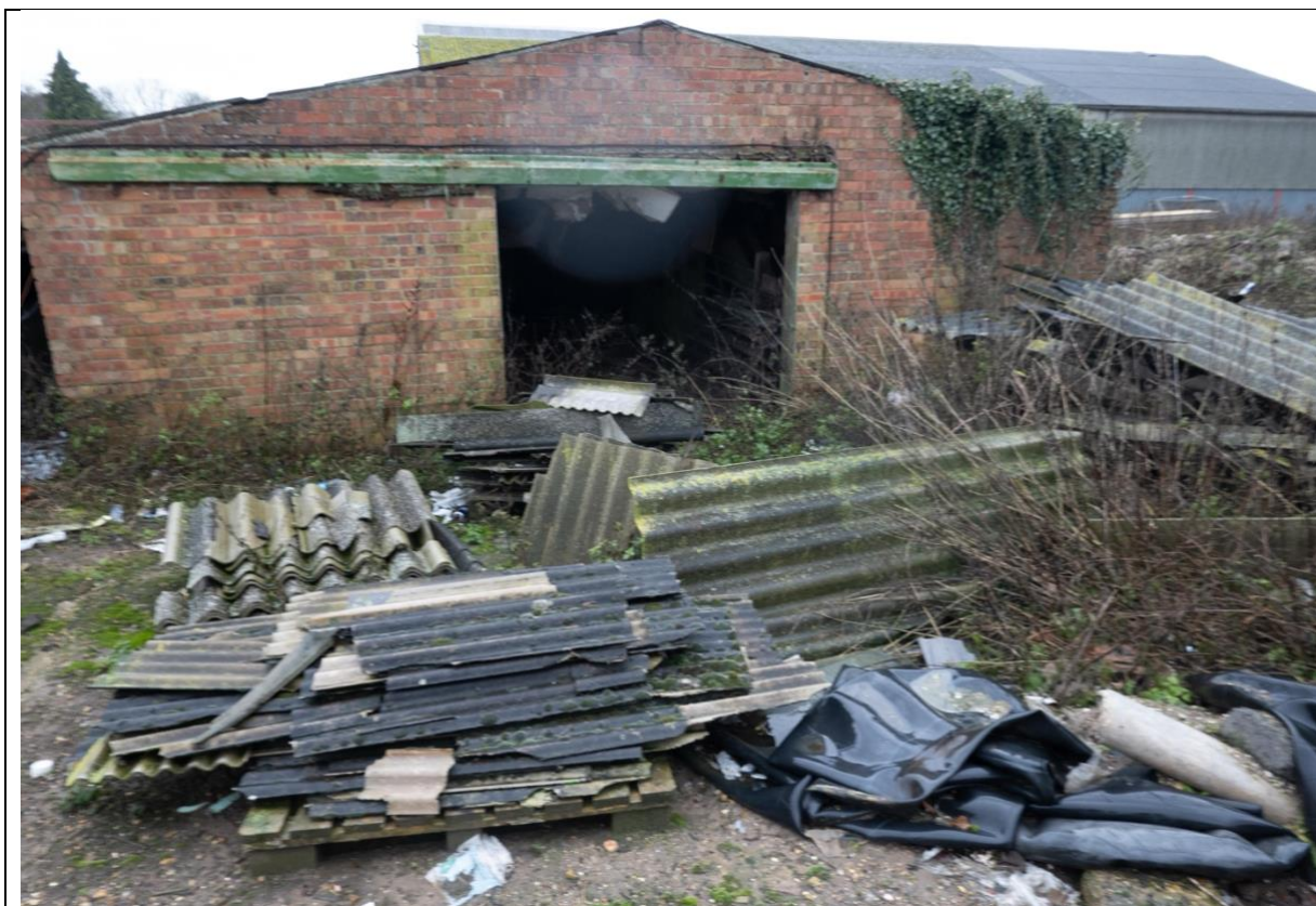
Figure 3.10 Asbestos roofing sheets adjacent to B2
