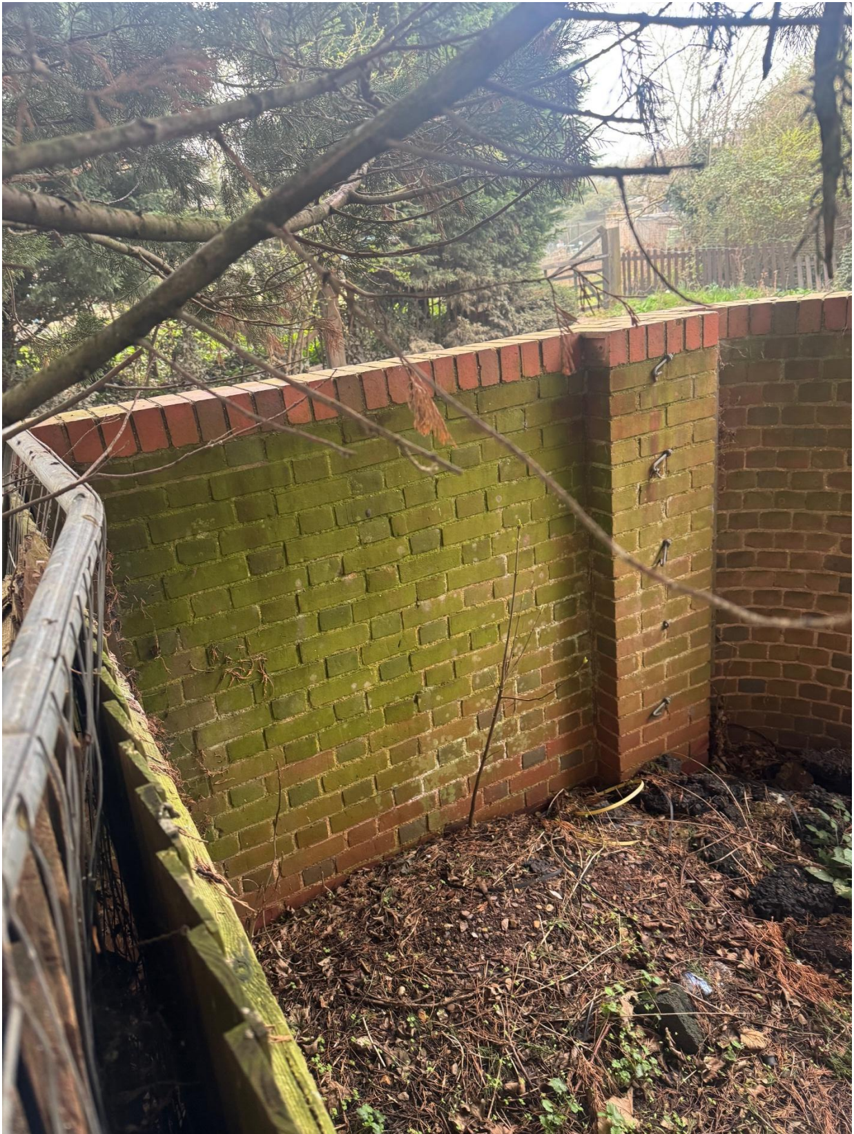
G1 – Wall in close proximity to Leyland cypress group
