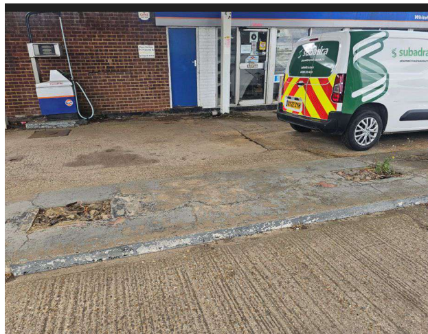
Photograph Five: Former pump island, with dispensers removed. Paraffin dispenser in background.
