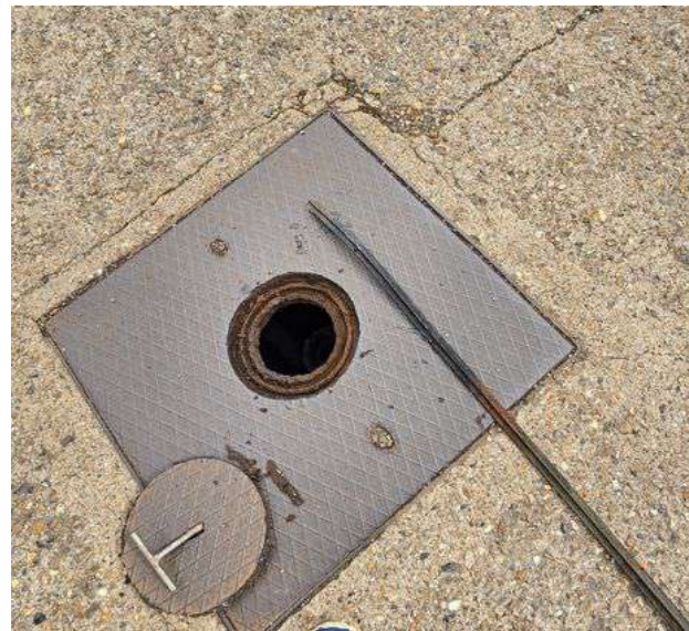
Photograph Nine: One of tank access chambers (direct fill point), with old dip-stick (used to measure tank contents). Small volume of water (no fuel) in base of tank.
