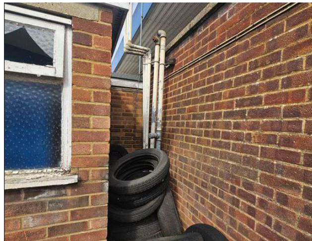
Photograph Seventeen: Former fuel vapour vent-stack. Five vents present, although two are labelled '6' and '7'. Waste tyres also present.
