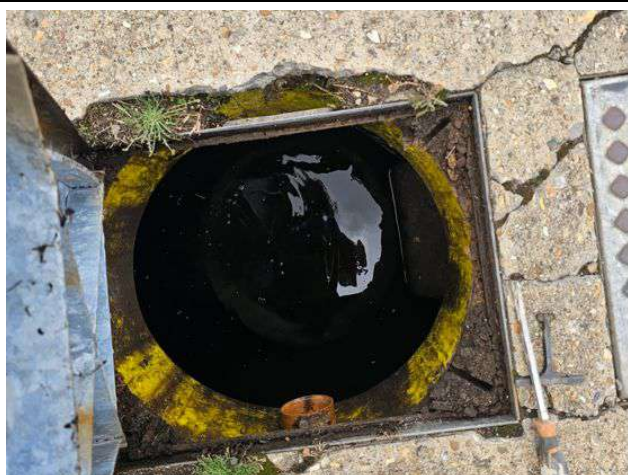
Photograph Ten: Forecourt interceptor, constructed from GRP. No fuel / oil evident.
