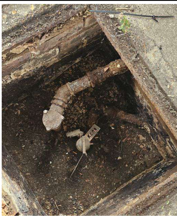
Photograph Seven: Inside of tank access chamber, showing metal fuel pipework.
