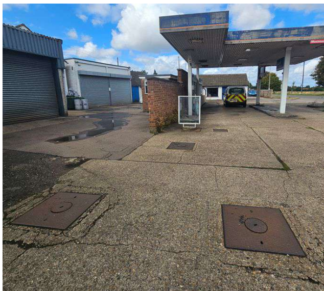
Photograph Eight: Main below ground fuel tank farm, at southern end of the site.
