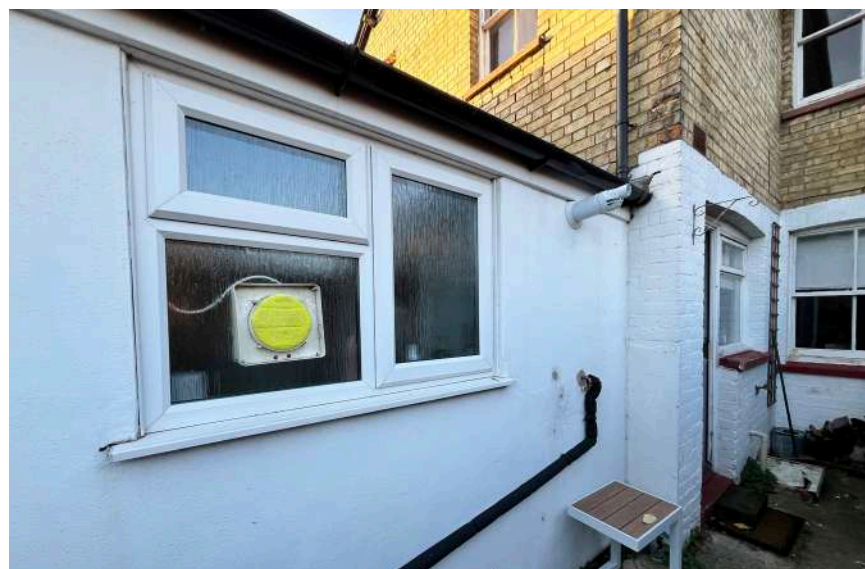
Existing extension and PVC window
