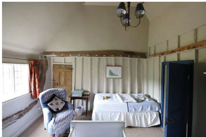
Photo of Bedroom 4 (looking west) in location of original 15th Century Medieval Hall, first floor insertion later addition. Small void above apex visible in loft space.
