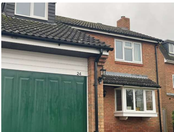
Photograph 5. Showing the slight lift in the wooden soffit.
