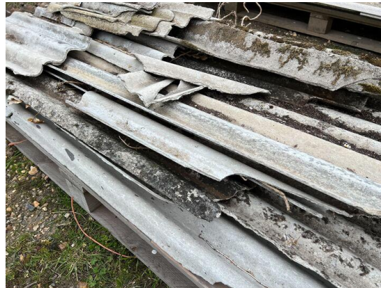
Potential asbestos sheeting.
