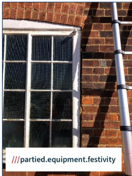
Figure 17. Missing mortar adjacent to window pane.
