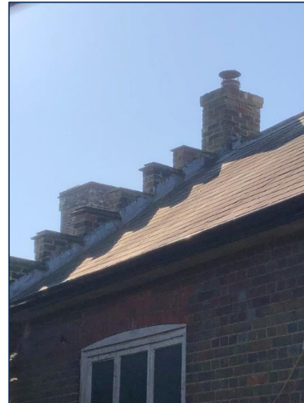
Figure 14. Lifted lead flashing upon cottage roof.
