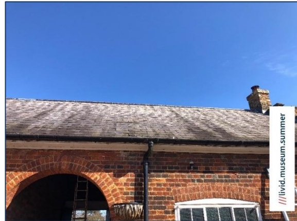
Figure 16. Multiple raised tiles along full length.
