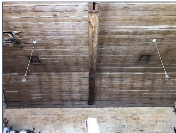
Figure 36. The rotten, wooden ceiling boards of the old stable.
