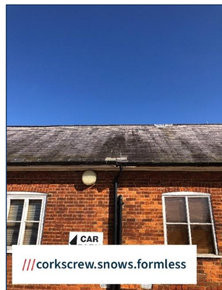
Figure 18. Slipped and missing tiles.
