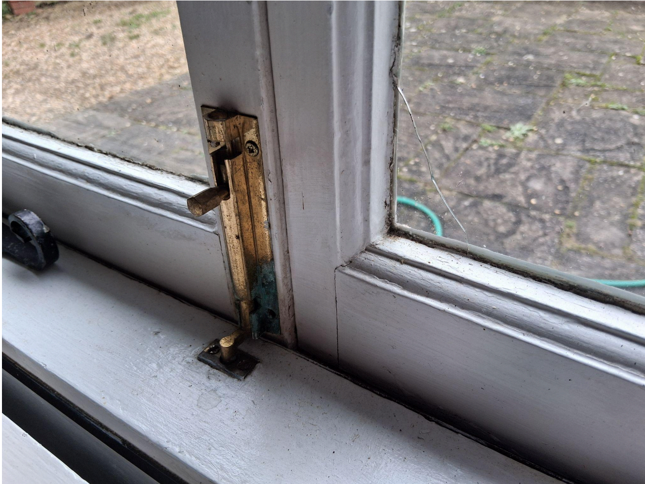
Window 5: Glass is broken and frame is warped so that window does not close tightly.
