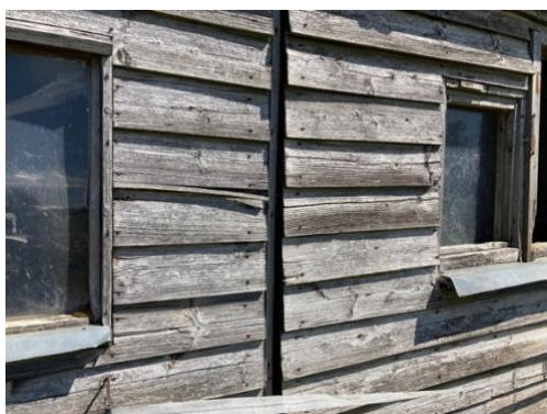
Photograph 11: Example of lifted wood cladding
