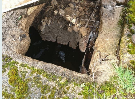
Flooded underground cavity
