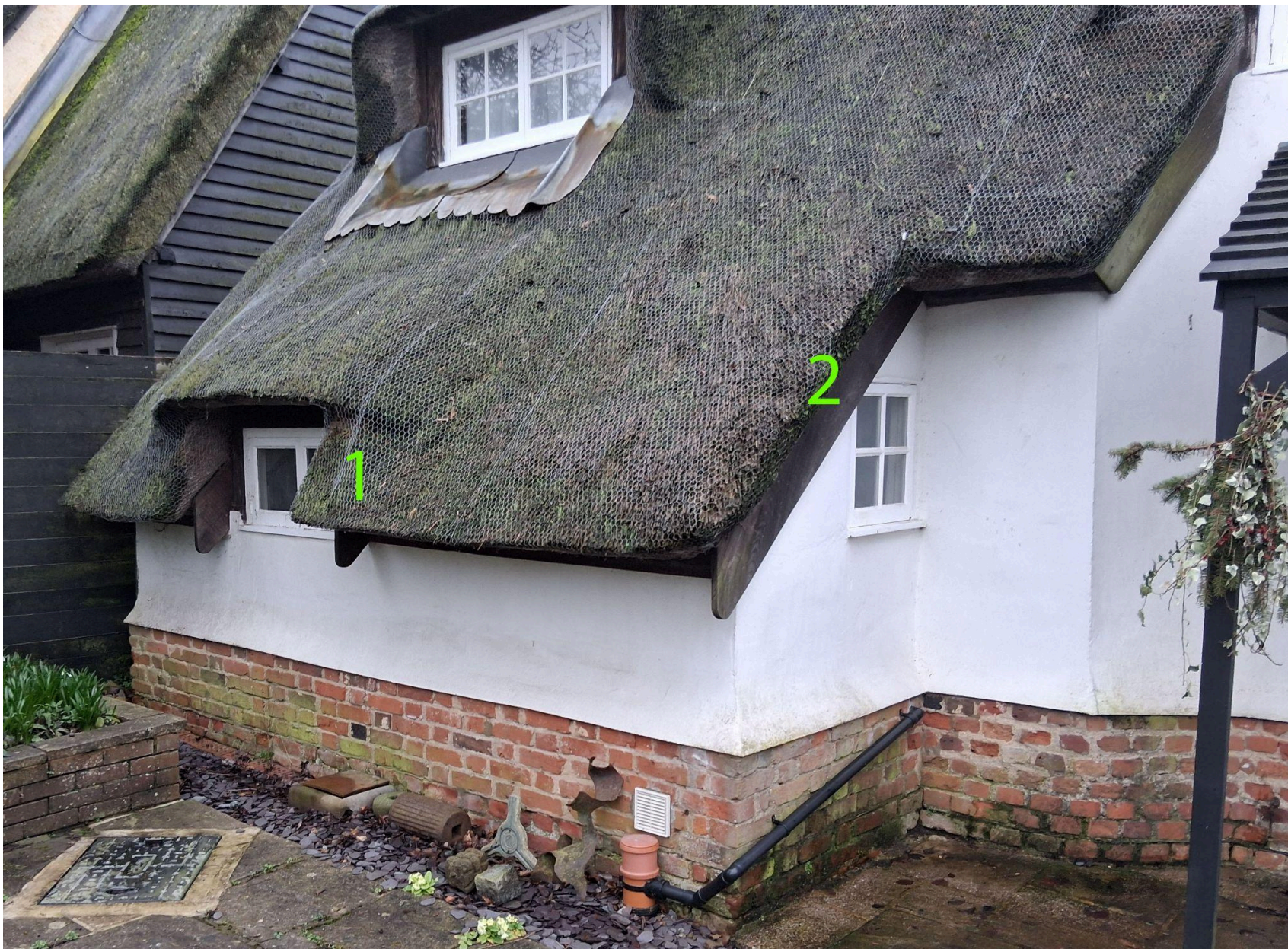
Rear_04: Bathroom(1 & 2) windows to be replaced.
