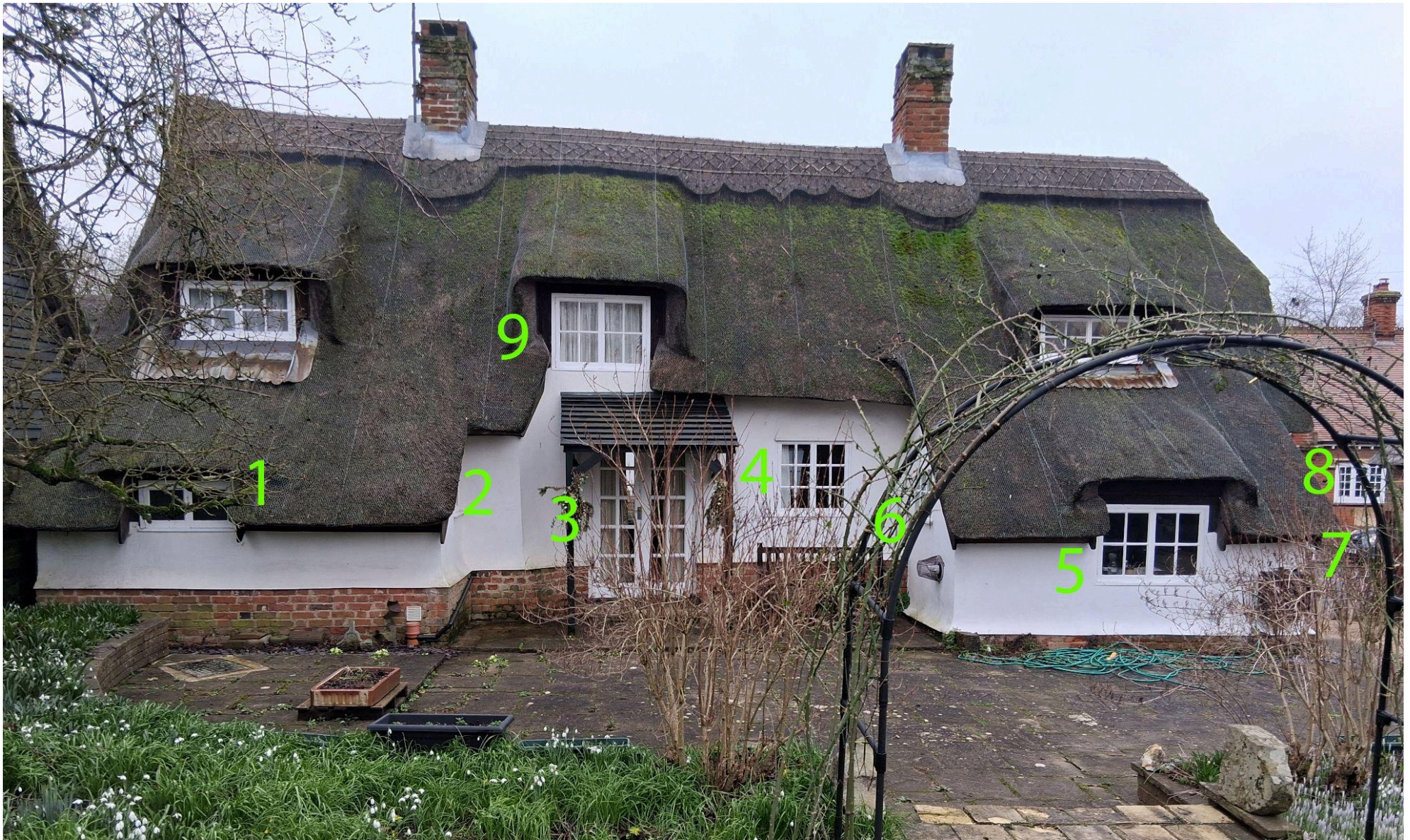
Rear_01: Nine windows on the rear and side of house to be replaced.
