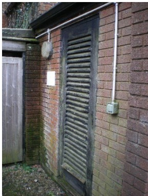
Feature 3: Ill-fitting and slatted door in a brick shed
