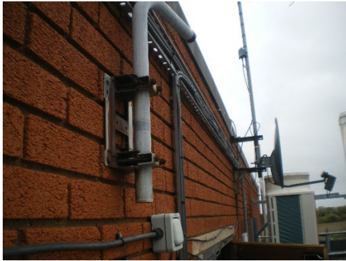
Feature 1: A long metal lip folded over the top of the wall from the roof. North west elevation
