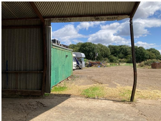
On the east side of the barn, the frame is impact damaged and the horizontal metal cladding frame missing.
