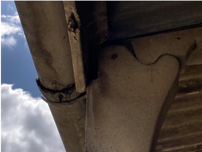
Some purlins have moved from their original bearing position and are at risk of falling.
