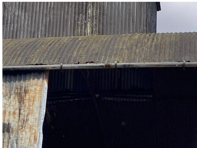
To the southern edge of the roof at the east end, the roof sheets are badly corroded and have partly broken away.
