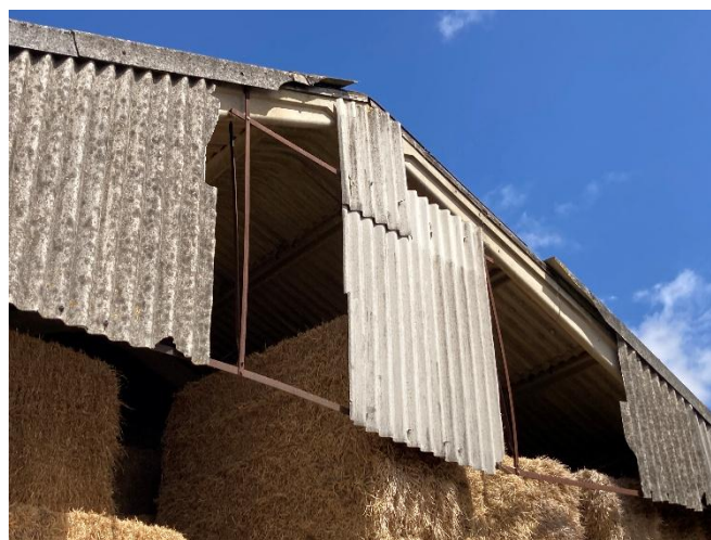
The cladding to the south gable end of the duo pitched roof is in poor condition and in danger of collapse.
