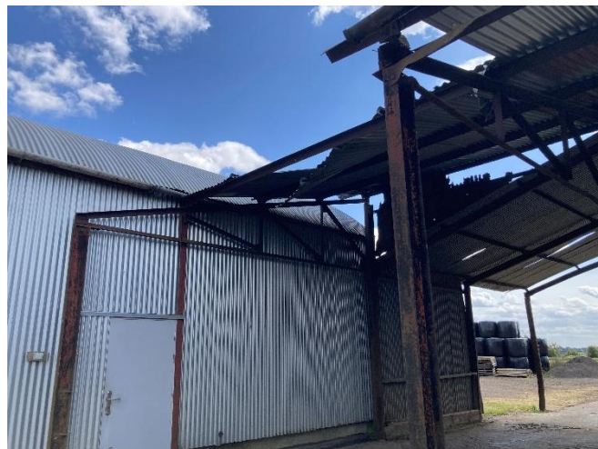
At the east side of the northern edge of the barn, a number of the roof purlins are missing.
