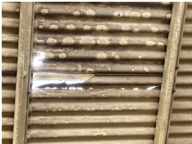
Some of the cement roof sheets are damaged, creating a safety risk and allowing water to ingress into the building.
