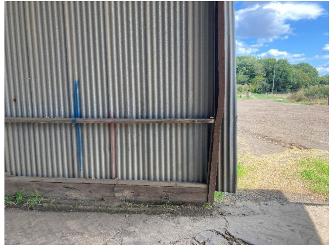
To the east side of the building, the central beam is impact damaged and bent.
