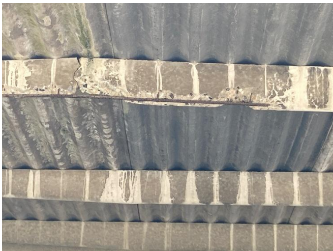
Many of the purlins have cracked and are in danger of collapse.
