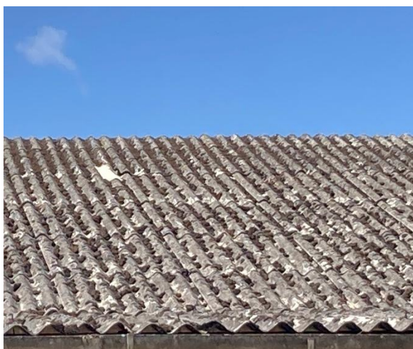
The roof has been patched repaired to a basic standard in sections. Repairing roof sheets that contain asbestos creates safety issues.
