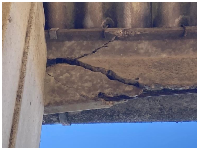
The concrete purlins have cracked and could collapse.
