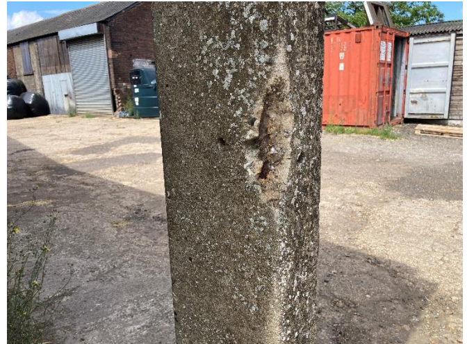
The concrete posts have localised areas of corroded reinforcement and cracking.
