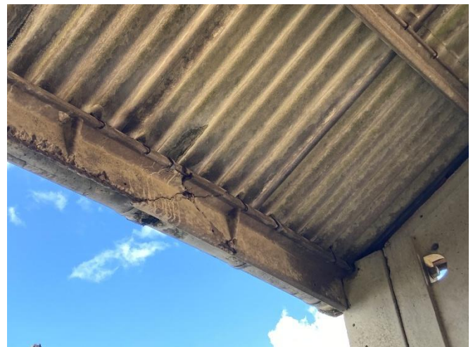
Some sections of the concrete are loose and could fall.
