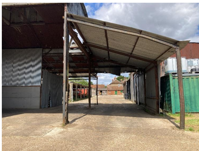
The diagonal steel beam at the east end of the southern perimeter of the barn is impact damaged.
