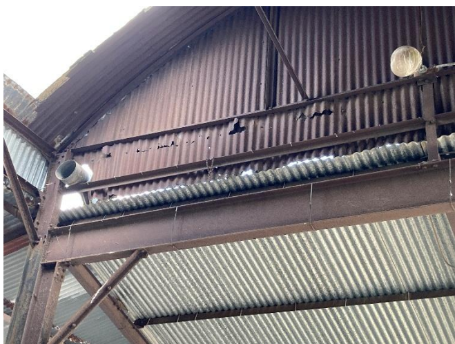
Vertical sheets in the barn, are badly corroded and have holes present in the sheets.
