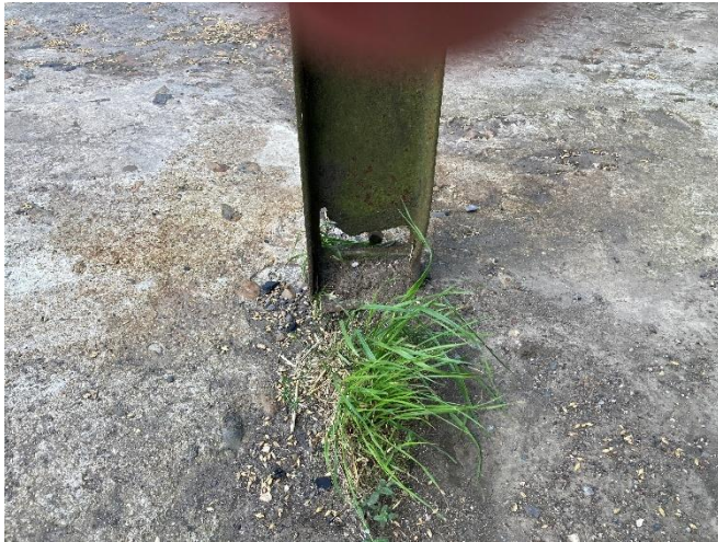
On the east side of the north elevation, the steel is badly corroded at ground level.
