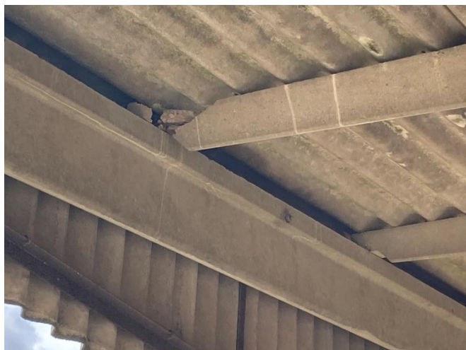
Some purlins are damaged where they bear on the beams.
