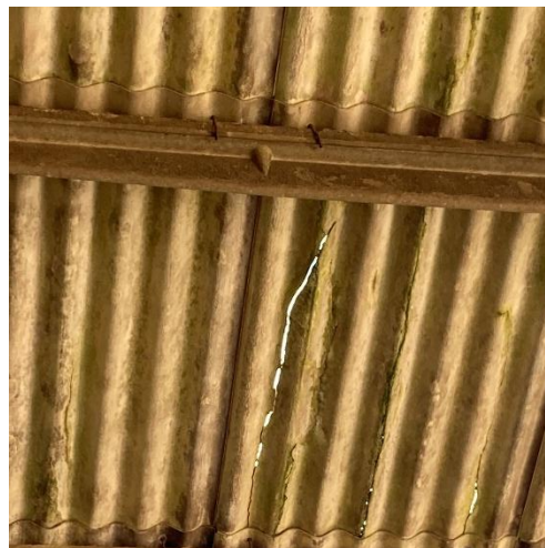
The roof cladding is cracked in sections.
