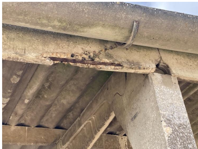
The reinforcement has corroded in sections, causing the surrounding concrete to become displaced.
