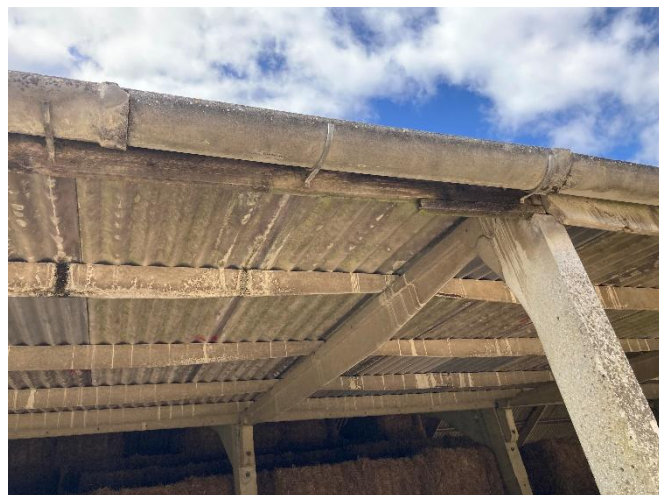
One damaged concrete purlin has been replaced in a basic manner with a timber purlin.
