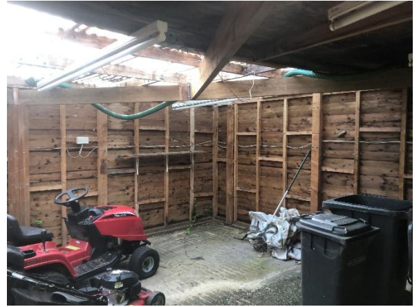
Plate 8: Interior of existing garage showing unsuitable light levels
