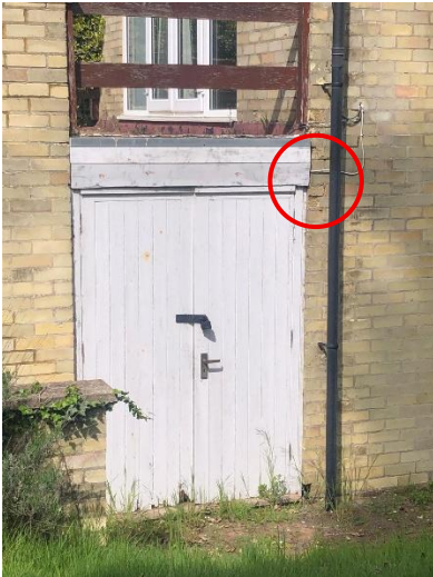
Plate 18: Gap in brickwork next to door frame, containing a blue tit nest
