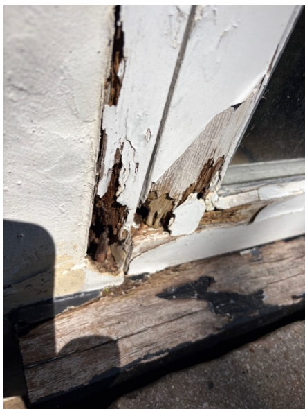
Photo 2: Close up of decaying frame and door, showing a state that is beyond repair
