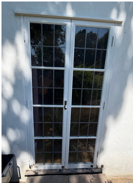
Photo 1: One of the two existing French door sets. The glazing bars match nothing else on the house; the glazing is single; the putty has failed; the paint and timber have broken down at the foot of the frame; and a rough, replacement cill has been installed at an unknown point in the past
