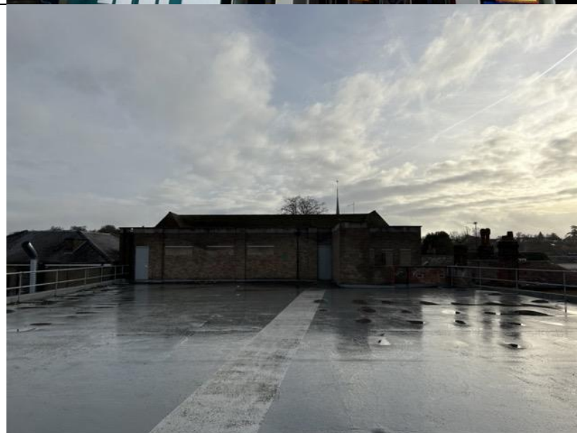
Photograph 2: Main section of the roof used as a car park (facing the high street)
