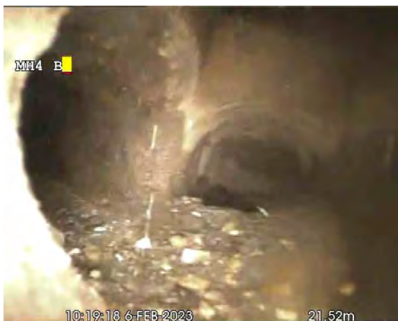
51395fd3-0329-4168-beb3-8c67e194c290.jpg, 00:01:44, 21.62 m Junction at 9 o'clock, 100mm dia
