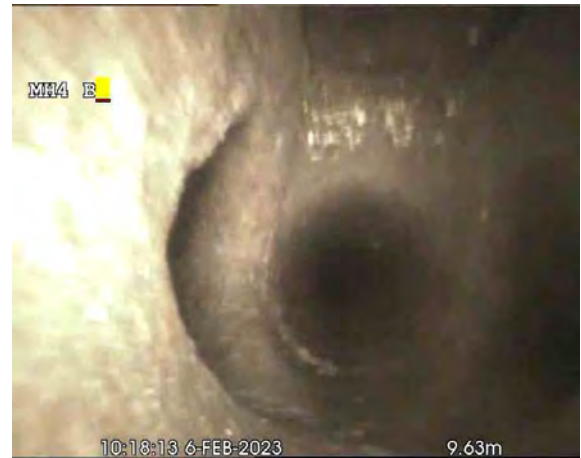
ee64899a-ccf0-4f8f-aebf-3013d63588b8.jpg, 00:00:38, 9.83 m Junction at 9 o'clock, 100mm dia
